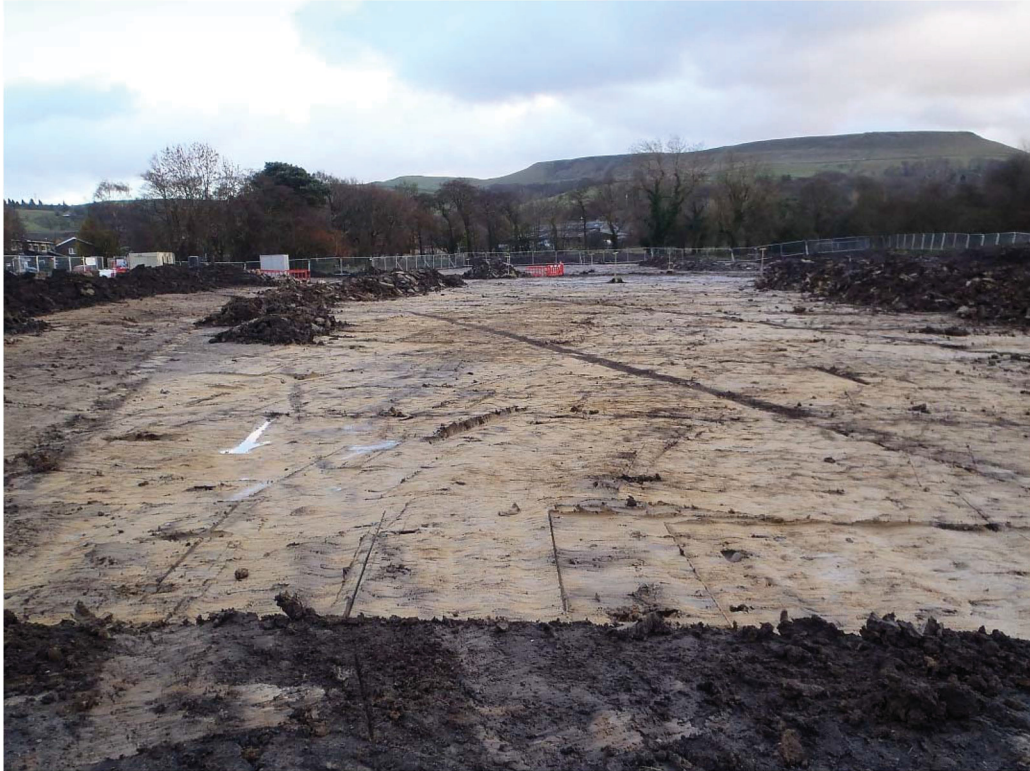
Plate 6: General shot of the site looking south once the cleaning was completed
