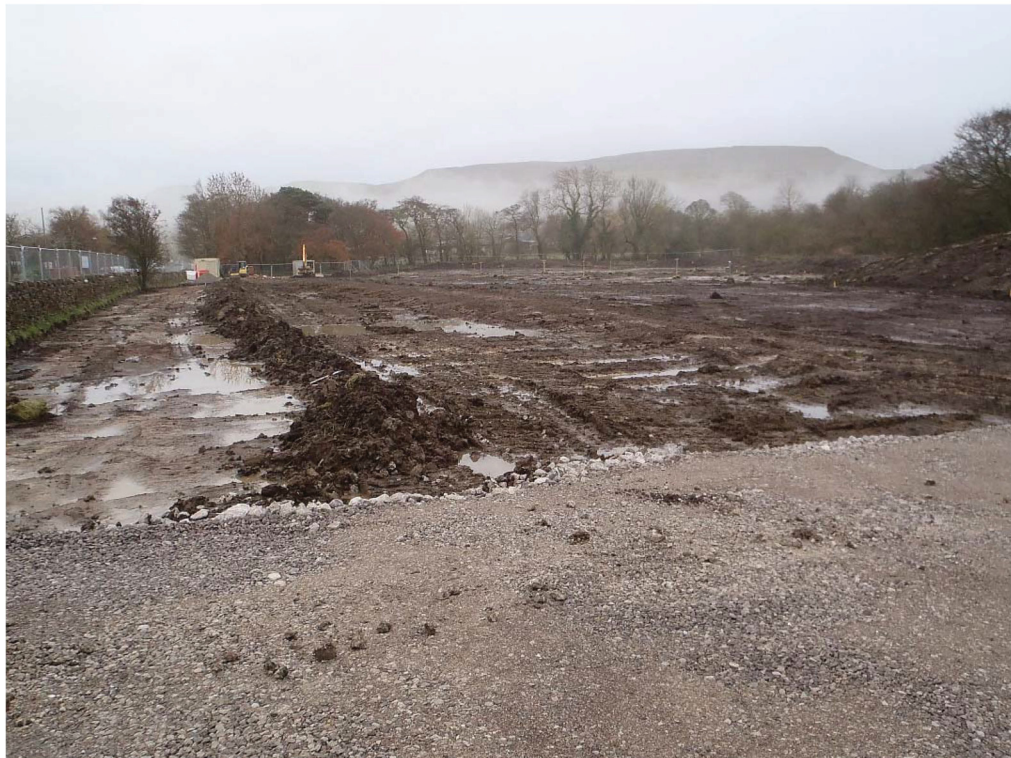
Plate 5: General shot of the site looking south, following stripping but prior to cleaning
