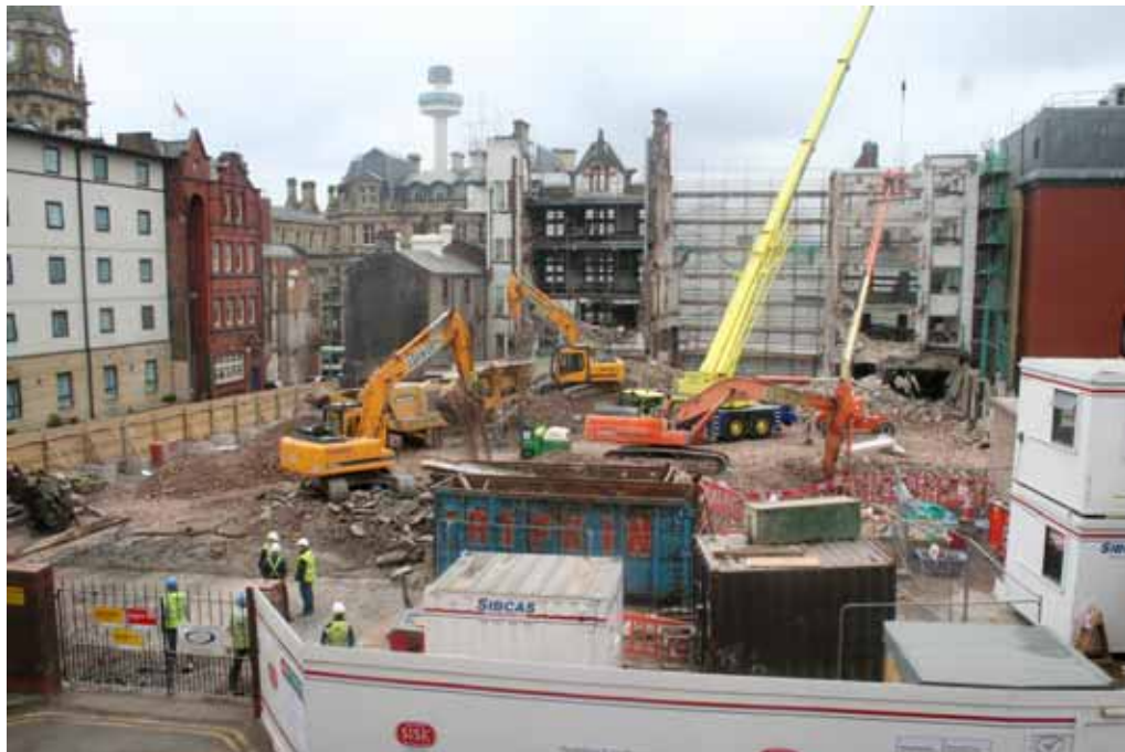
Plate 2: South facing view showing the excavation area in the foreground with ongoing demolition work of 57-65 Dale Street in the background
