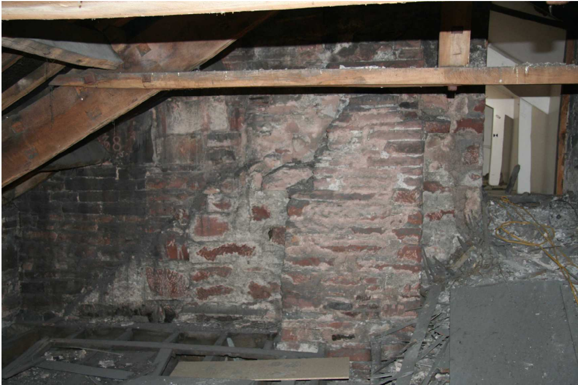
Plate 39: Wall scar, west elevation, room 32
