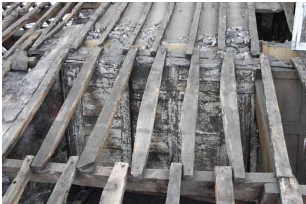
Plate 27: Section of timber panelling situated on the south side of the roof forming the south wall of Room 30
