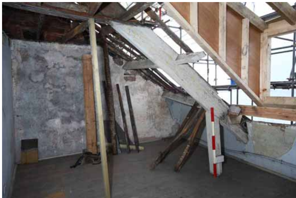
Plate 24: Example of a garret room (Room 30) in the central section of roof
