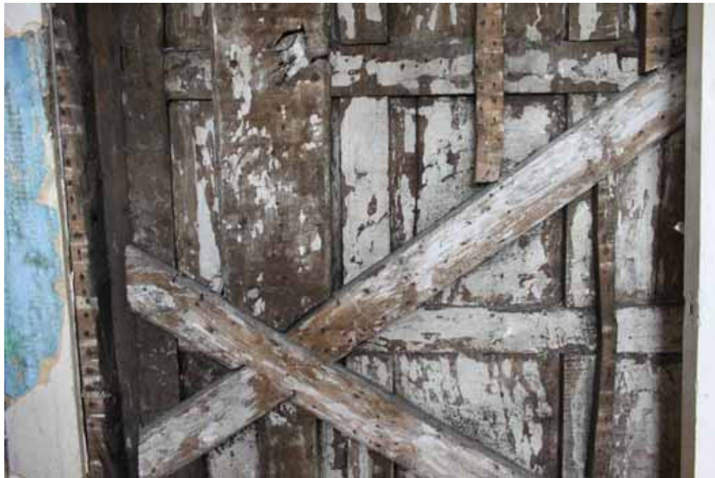
Plate 26: Detail view of the braces and upright member in the panelled wall
