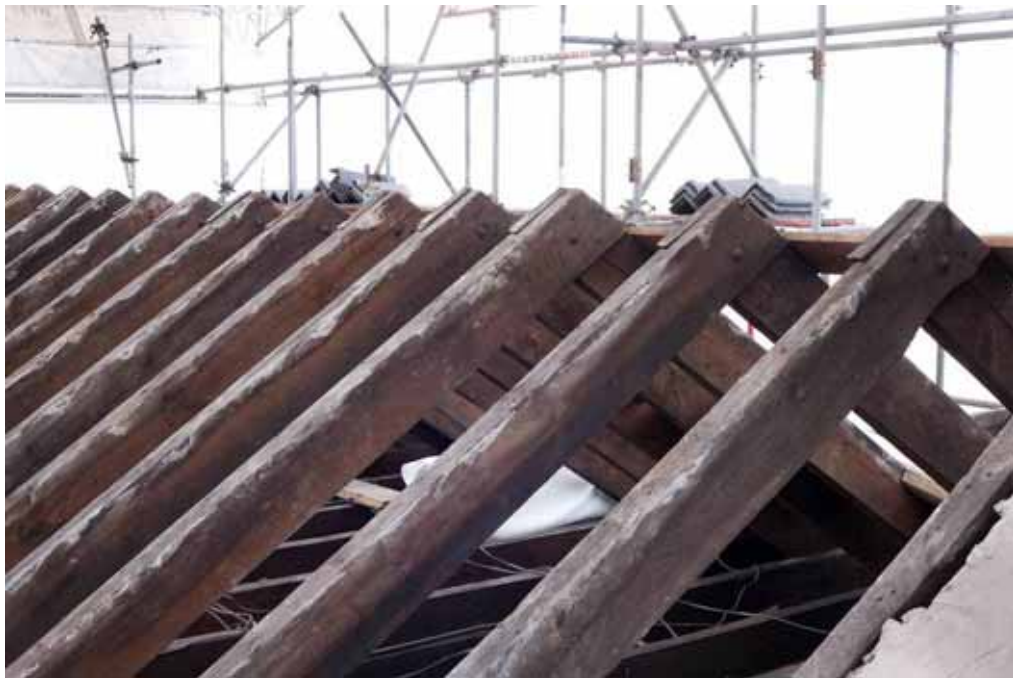
Plate 20: Detailed view of assembly marks on the trusses of the western roof
