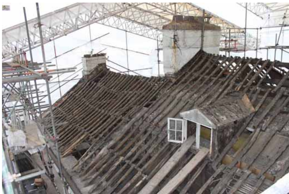
Plate 19: General view of the eastern and central sections of the roof, facing south-east
