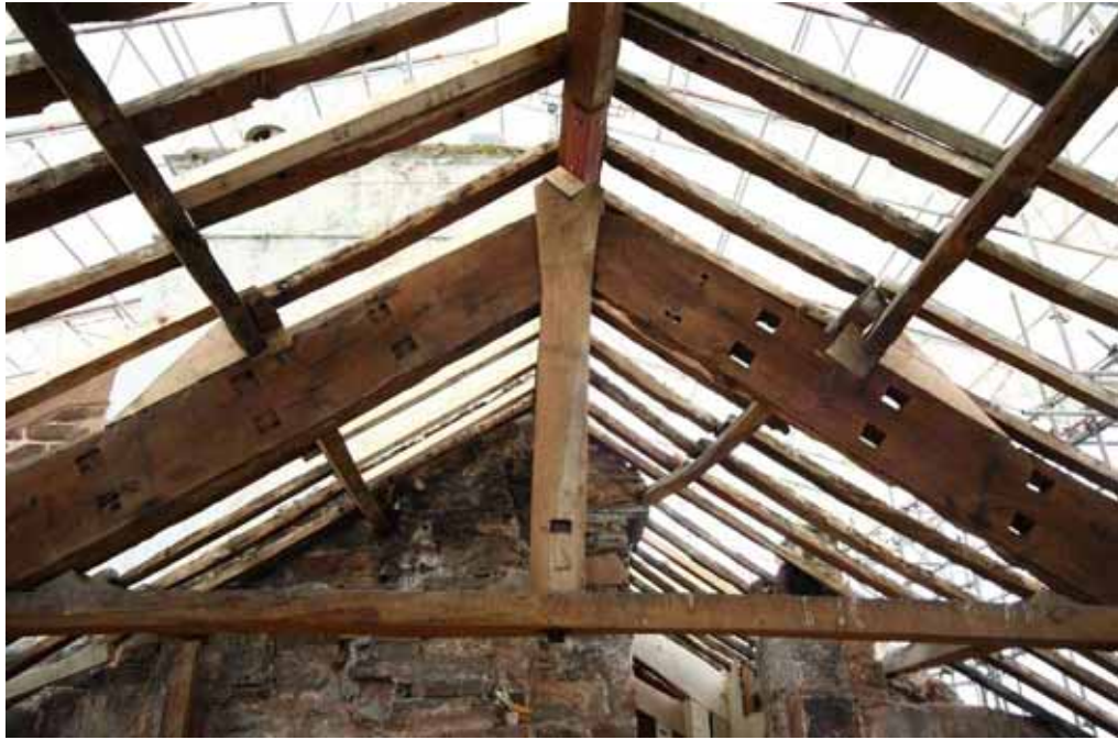
Plate 31: The west truss with holes clearly visible in the principal rafters
