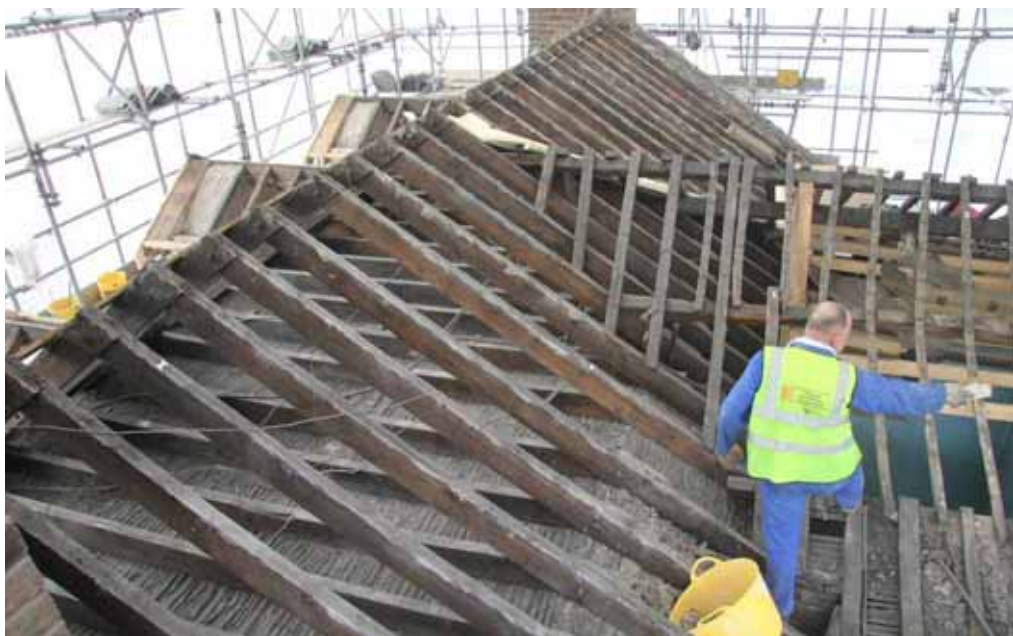
Plate 21: View of the join between the west and east roof sections
