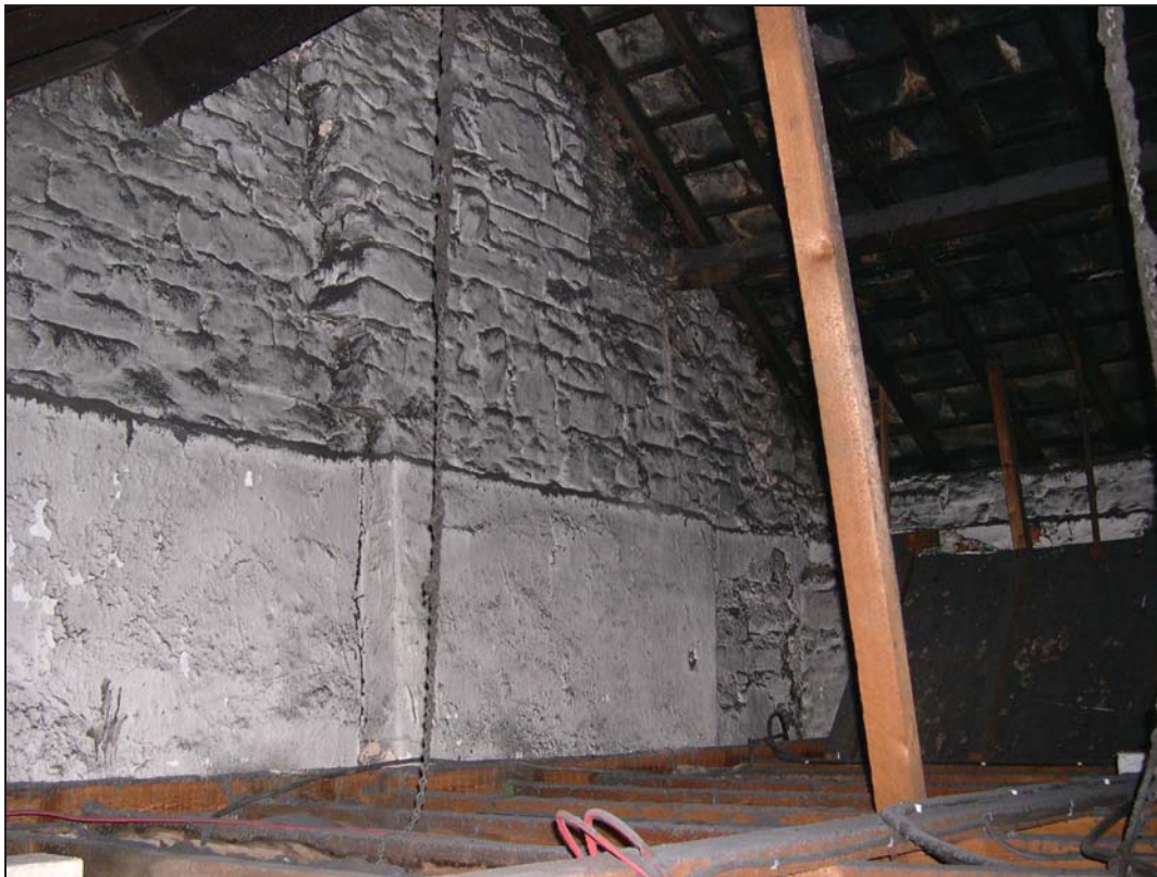
Plate 16: Scar in Space Above Room 2
