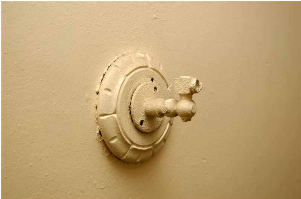
Plate 60: Gas fitting in Room U005
