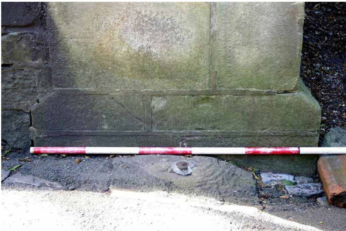
Plate 100: Example of the plinth at the base of the post, together with remnant of the gate hinges
