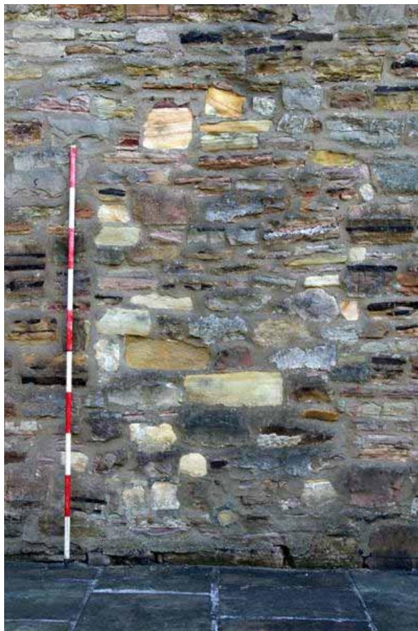
Plate 30: Possible blocked doorway in the north-west elevation of the Museum
