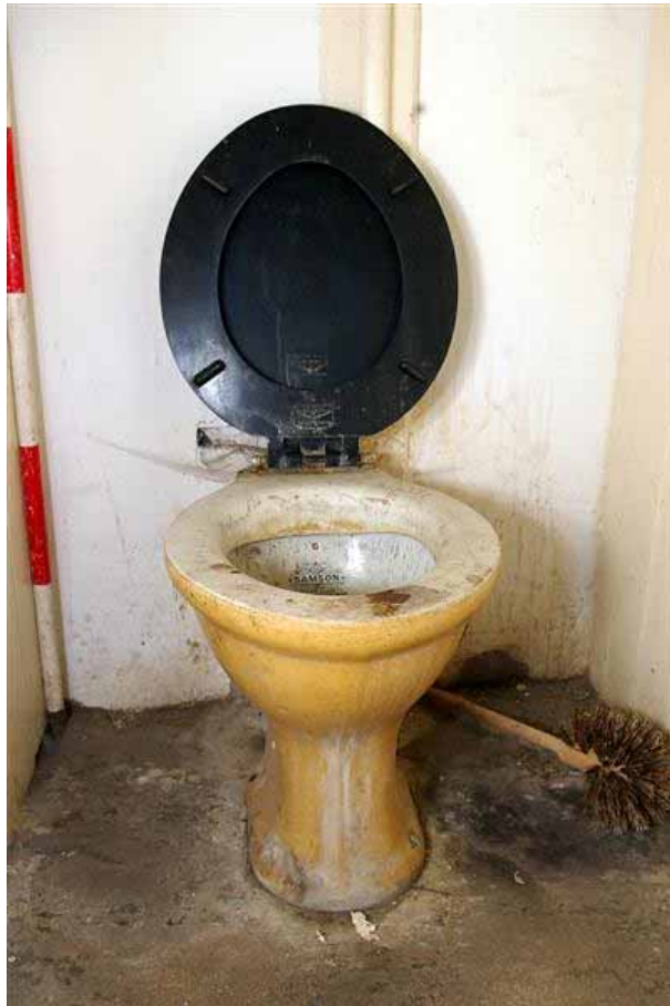
Plate 98: The 'Samson Wash-Down Closet' in Room L112 of the Court House
