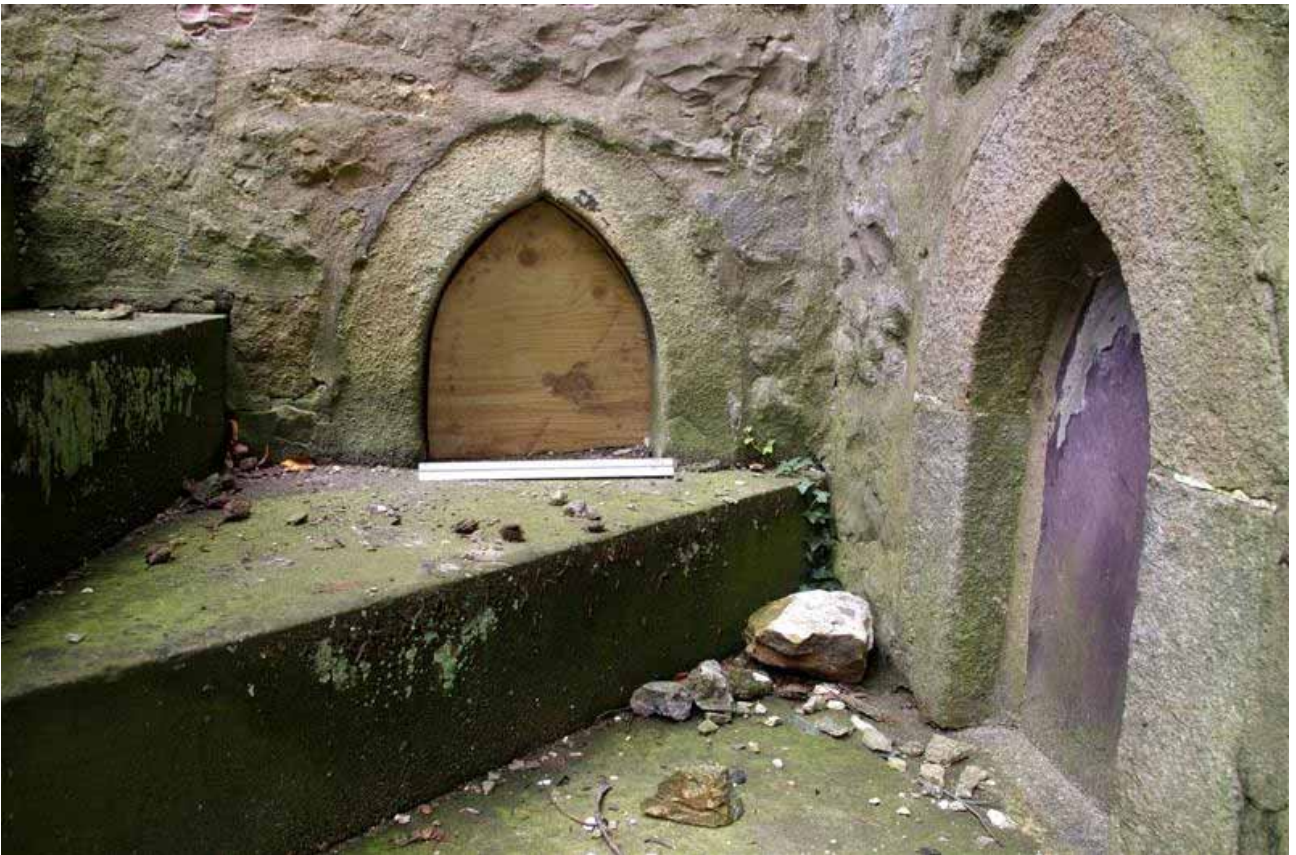
Plate 18: Blocked windows at basement level of the south-east elevation of the Museum
