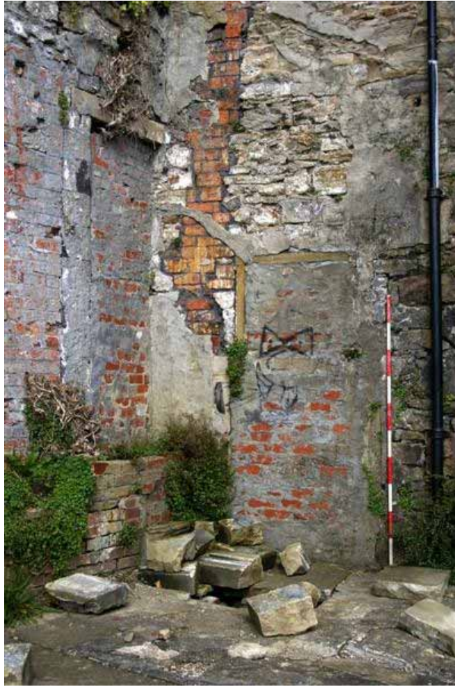
Plate 27: Blocked doors at the rear of the Museum building
