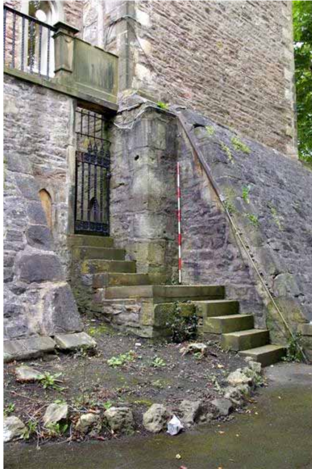
Plate 19: Steps allowing access to the balcony on the south-east elevation of the Museum
