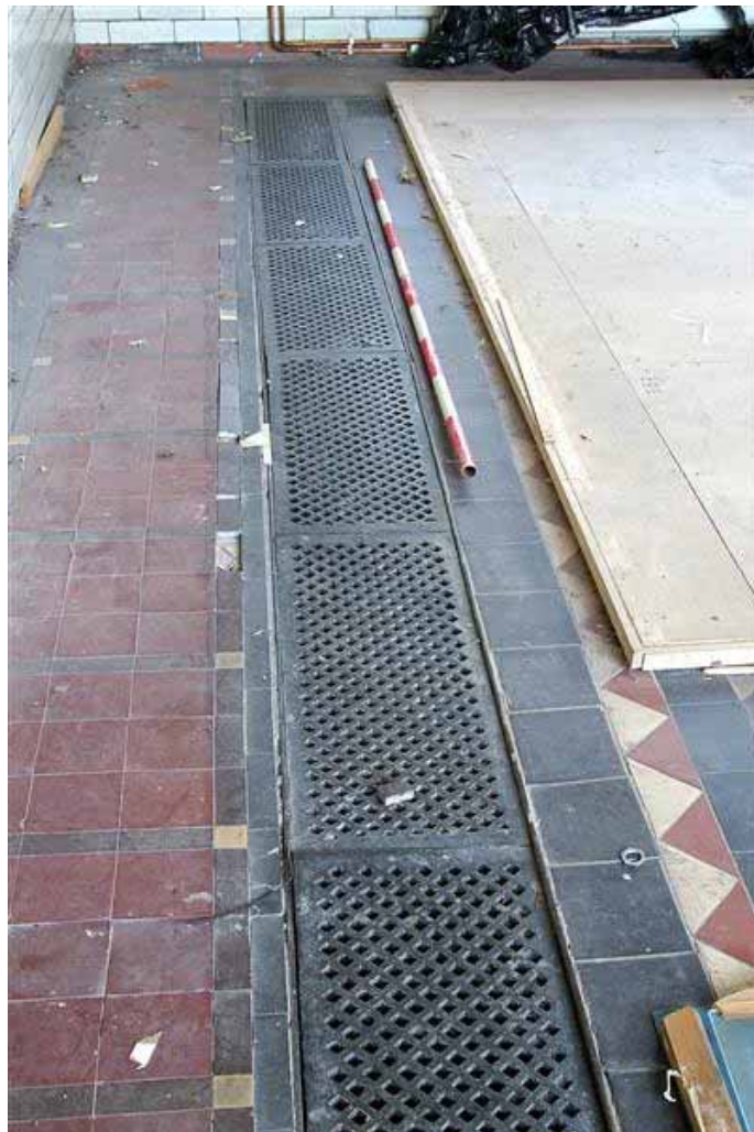
Plate 92: Heating grille in the floor of Room U107 of the Court House
