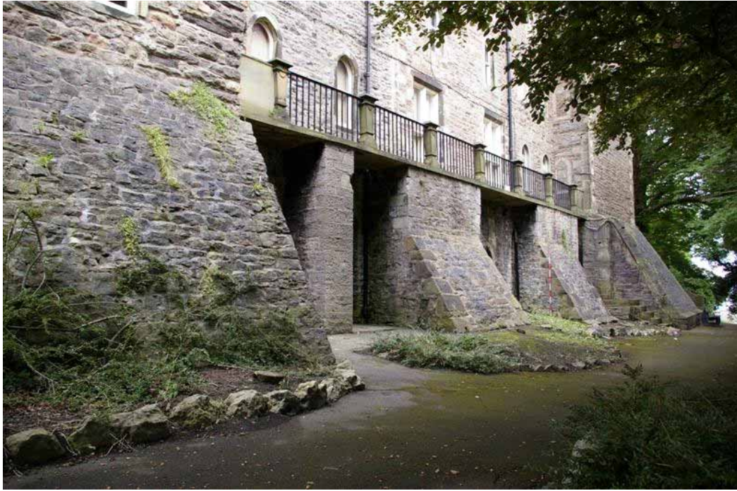
Plate 7: Buttresses and balcony at the base of the south-east elevation of the Museum
