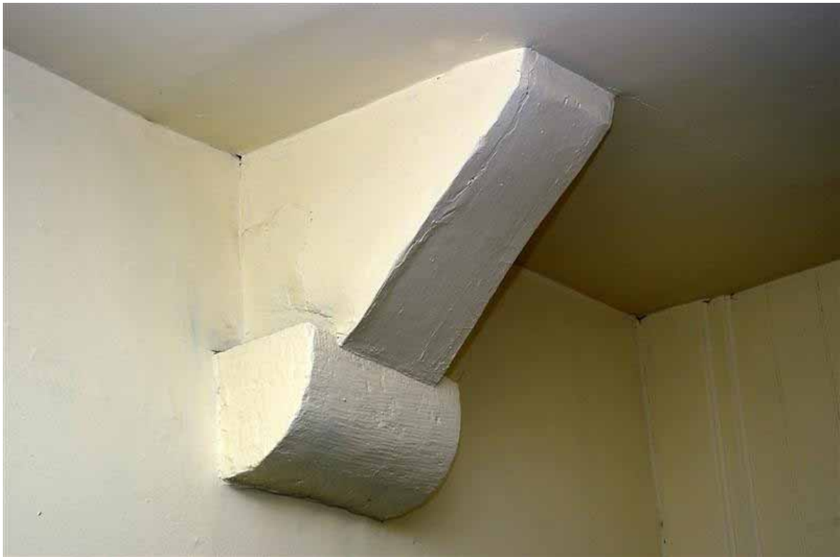
Plate 84: Corbel and base of truss in Room U102 of the Sound Archive
