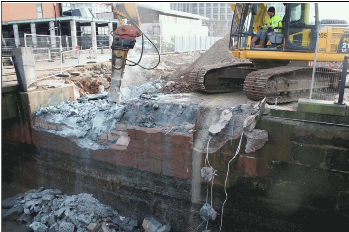
Plate 8: Princes Dock: the south wall during demolition, showing the materials used when the wall was reinstated in the 1980s
