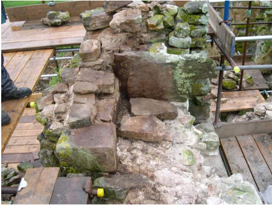
Plate 15: Sandstone jamb and passage to the parapet-level garderobe, south elevation of the barbican
