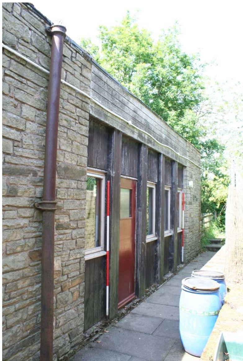
Plate 10: Detail of windows and door with wood-clad surround on the east-facing elevation of the communal part of the 1960s YHA building
