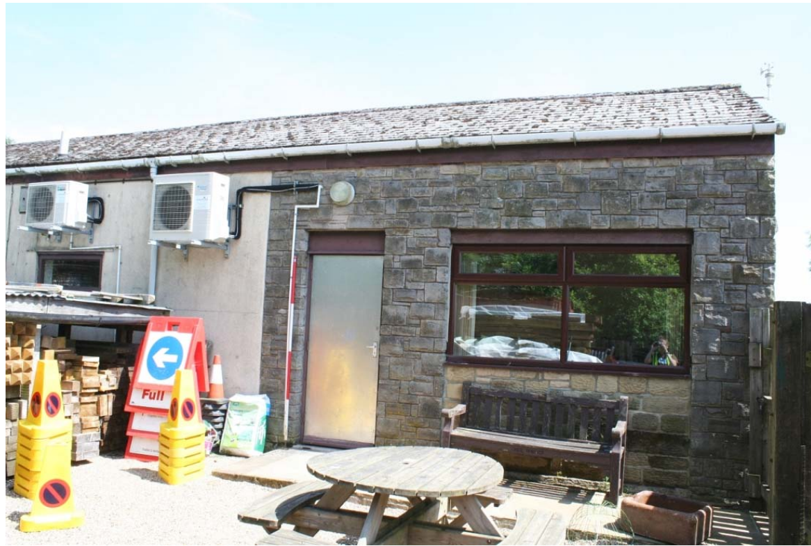
Plate 18: The exposed section of the east-facing elevation of the NNPA Visitor Centre, on the west wing
