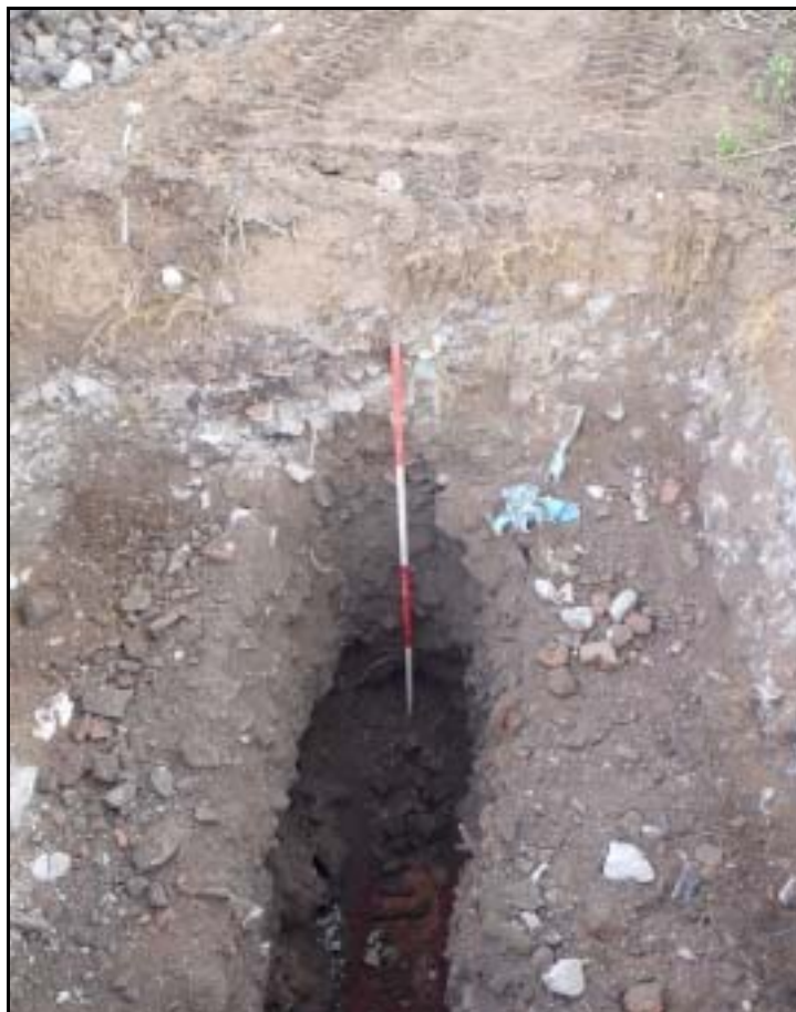
Plate 6: Trench 5, facing west, with the machine-cut sondage through the modern deposits to expose the natural bedrock
