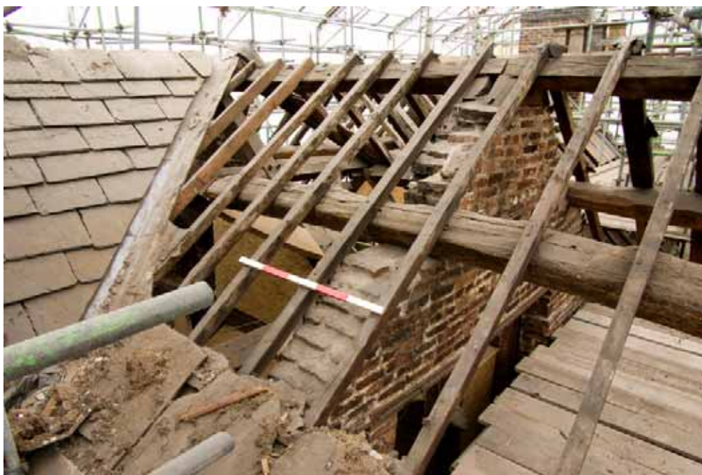
Plate 74: Timber saddles below butt-jointed ridge purlins, and redundant lap joint in purlin below, Roof L
