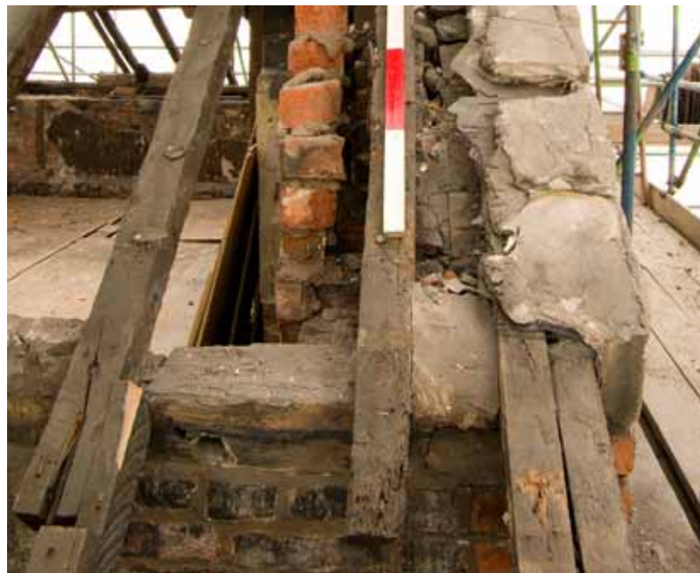
Plate 72: Bridled scarf joint in wall-plate, adjacent to north gable, Roof J
