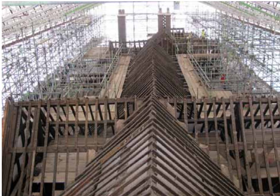
Plate 62: Aspect of roofs from west. Note bridled scarf joints on ridge of transverse Roof F
