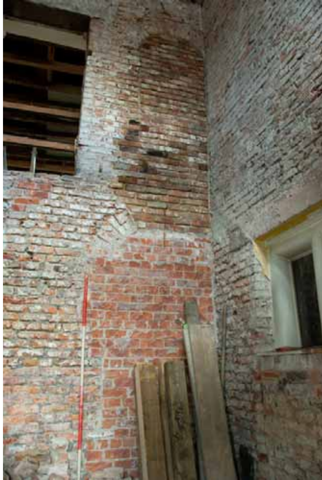
Plate 24: Blocked doorways in the Stair Tower, at ground and first floor level
