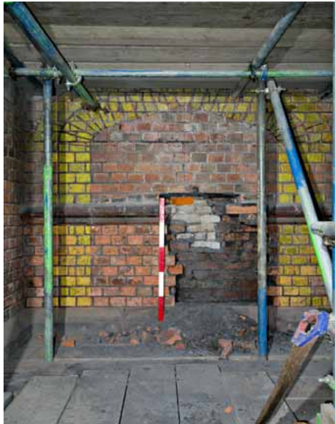
Plate 6: South external wall of the Great Hall (G4), showing the position of the new doorway
