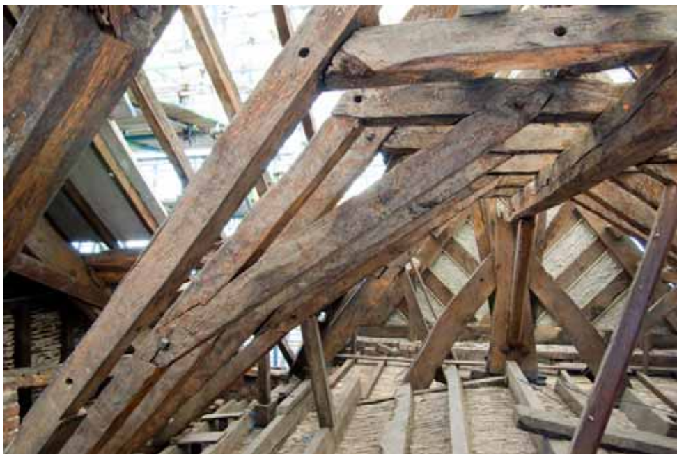
Plate 47: South truss, with detail of rafter, collar, and soulace construction, Roof C
