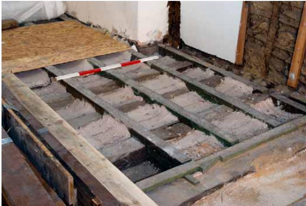
Plate 34: Later joists associated with an extension to the south of the Great Chamber, notched over the earlier fabric
