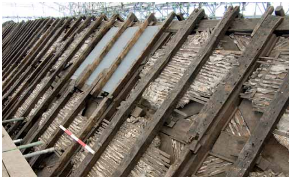
Plate 56: Blocked louvre, southern pitch, Roof D
