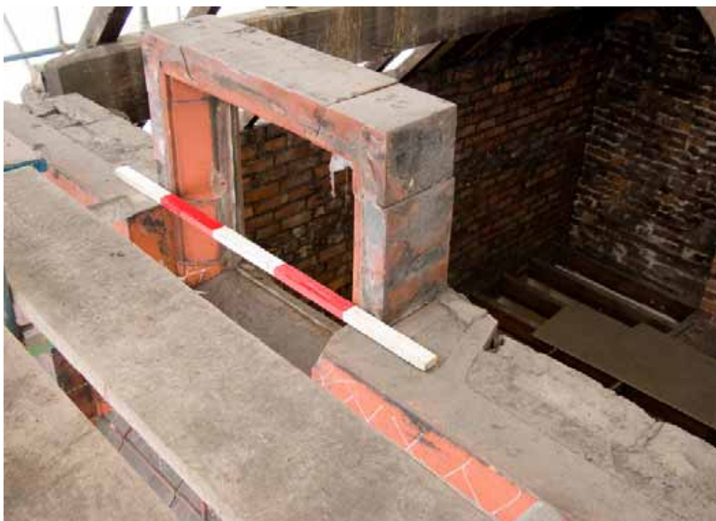
Plate 70: Joggled terracotta window surround, with maker's stamps 'O.H.' and 'AX' (Roof I)
