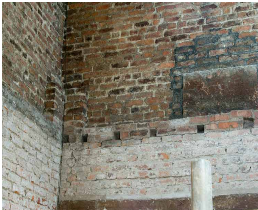
Plate 22: Reduced wall thickness at second-floor level of the stair tower
