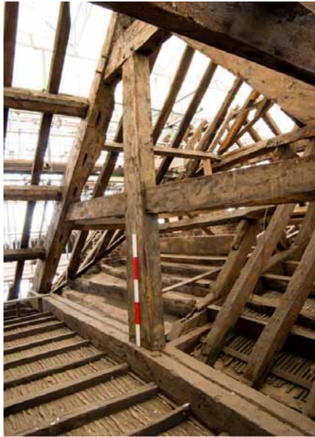
Plate 49: Eastern truss, Roof D, with scarfed common rafters of Roof C behind (bottom right)
