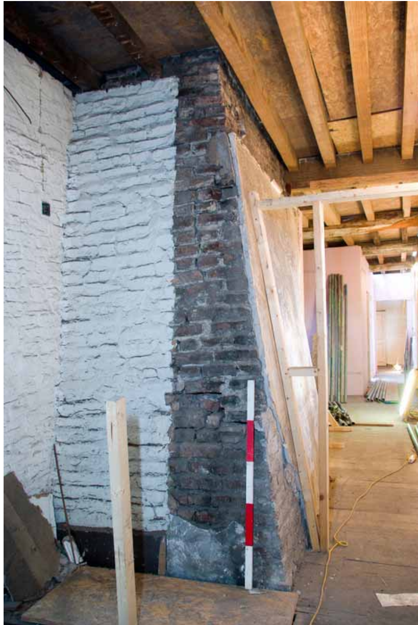
Plate 32: Chimney-stack revealed by removal of a later wall in the Egerton Gallery
