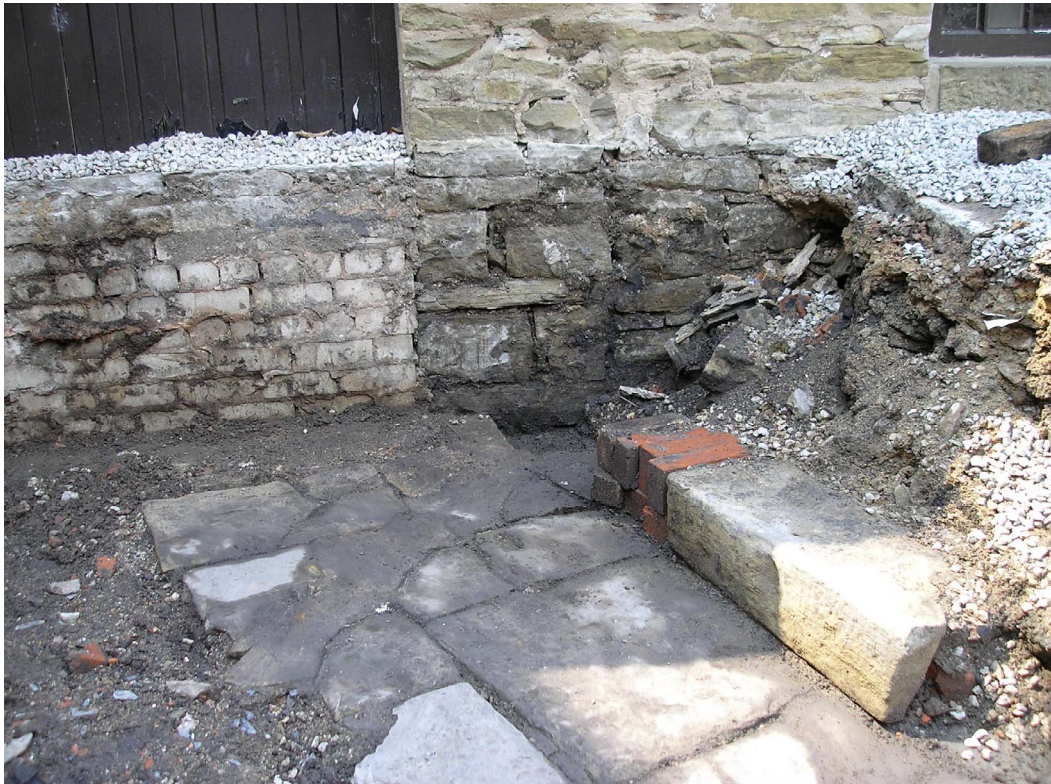
Plate 6: Boiler house floor, Trench A, with east wall of 1980s extension to the rear
