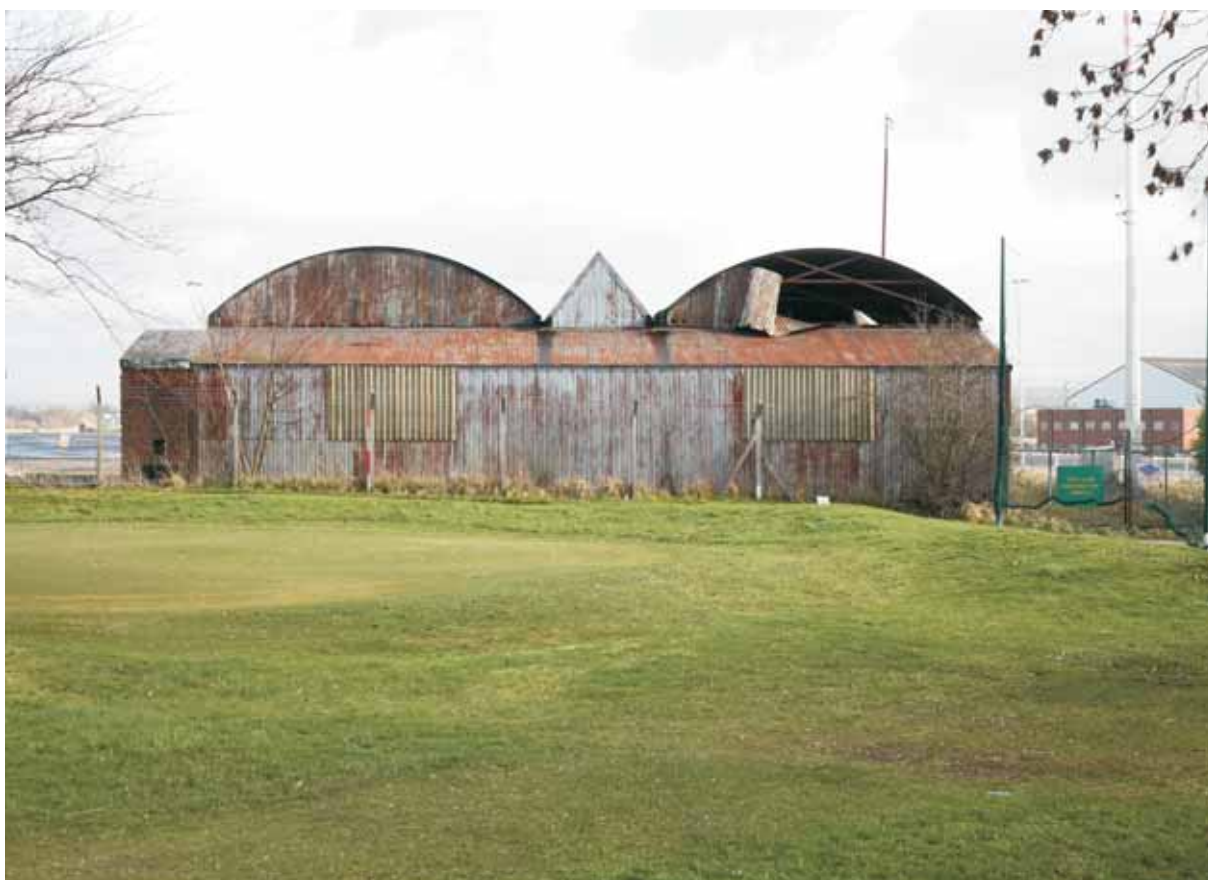
Plate 10: Rear south-west facing elevation of the Avro Shed, showing the full width lean-to
