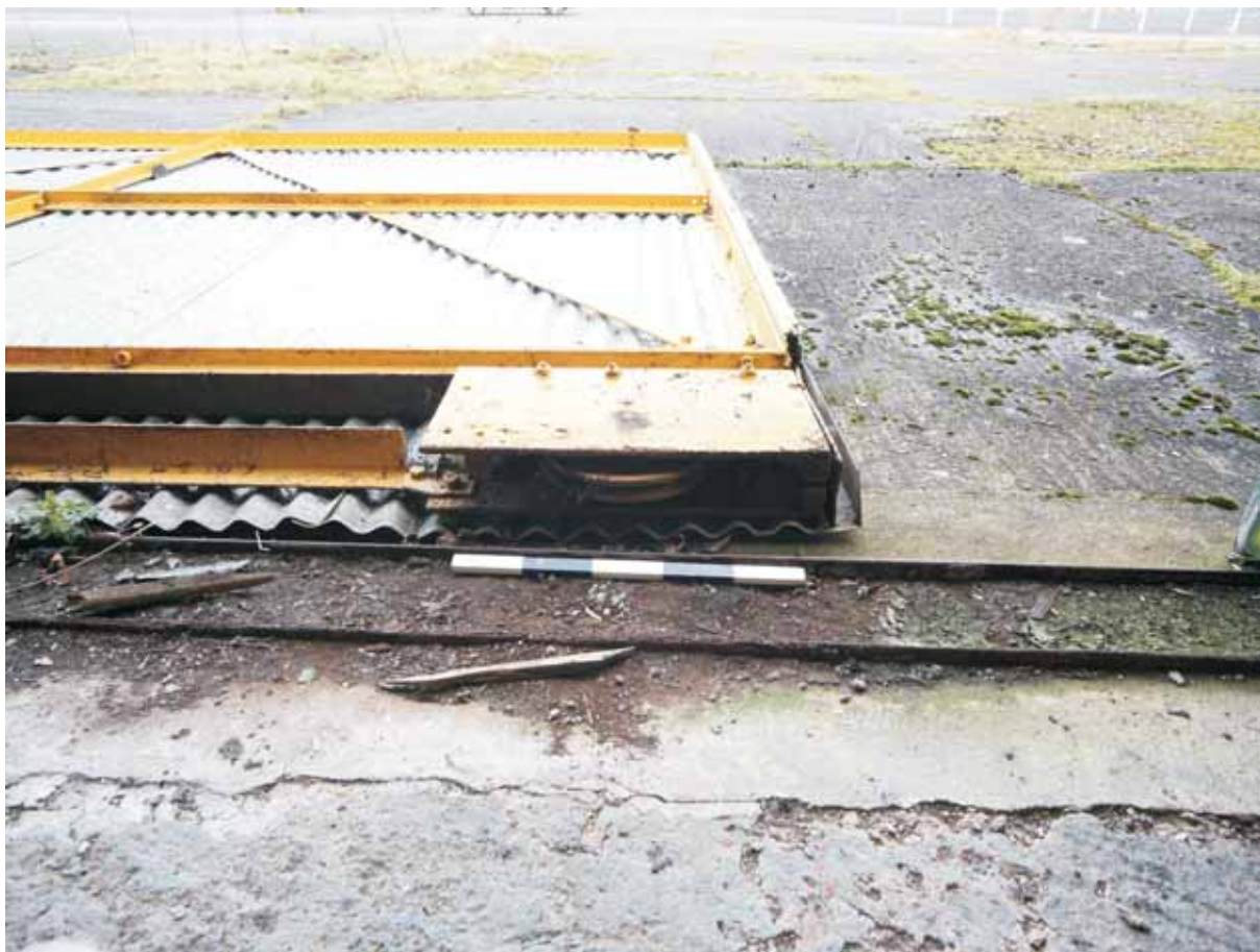
Plate 15: View of the roller on the bottom of the fallen sliding door, and the inset rail
