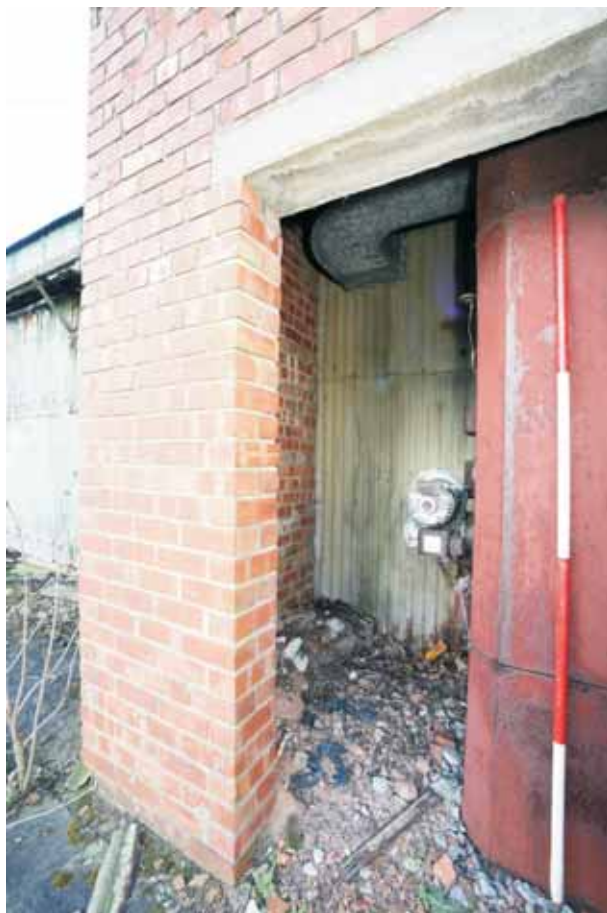
Plate 39: Boiler and heating duct visible within the brick outshut
