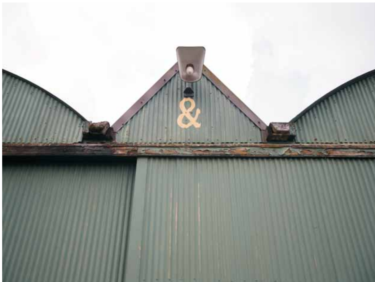
Plate 17: The pitched roof gable on the principal elevation showing the timber-channelled lead-lined gutters and angle-poised electric light
