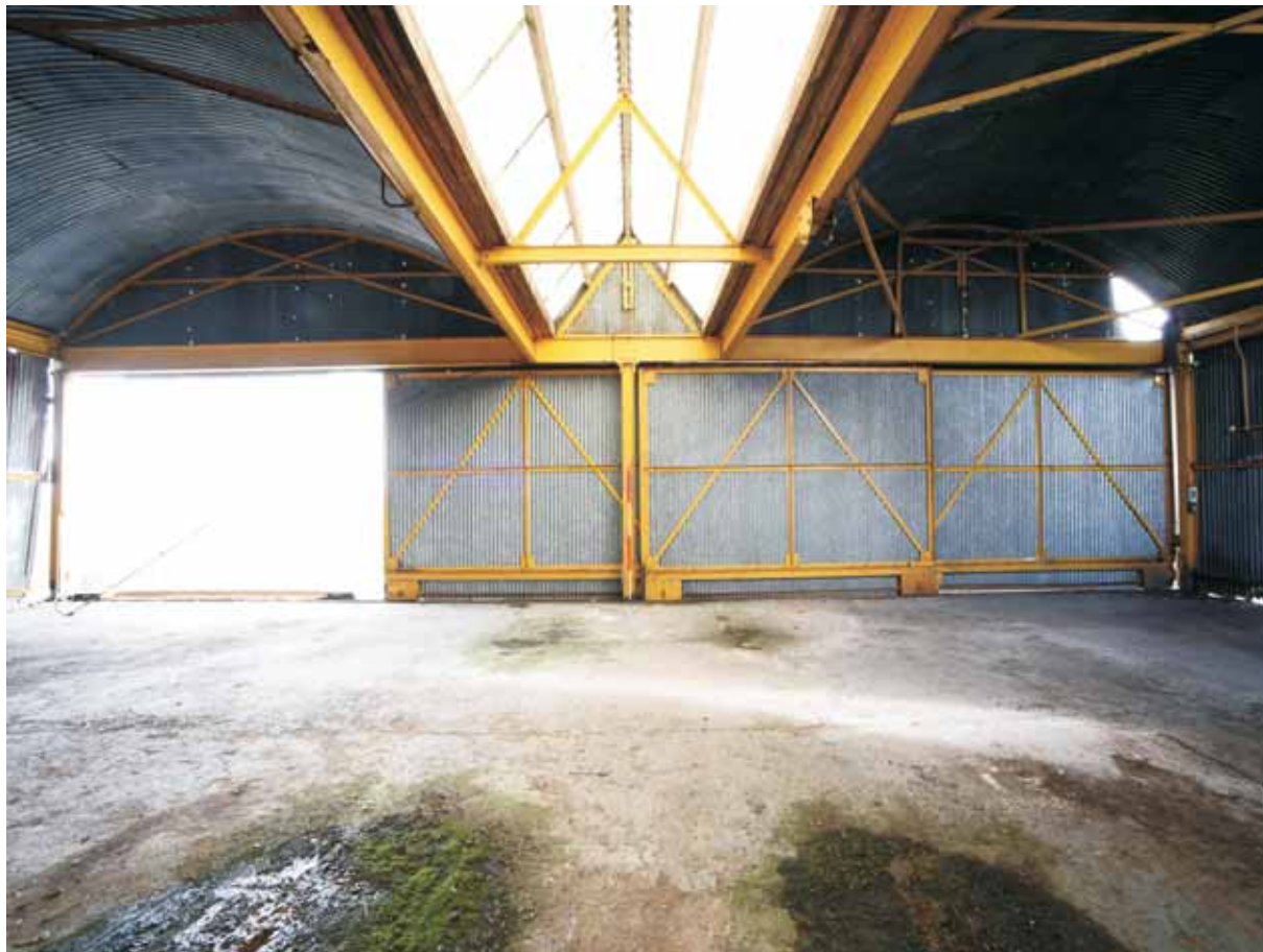
Plate 13: View facing north-east, towards the rear of the principal elevation, showing the roof trusses
