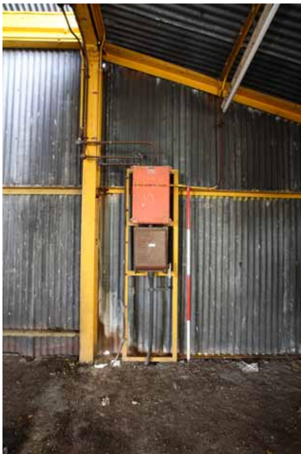
Plate 35: Fuse distribution box attached to south elevation, Room 1
