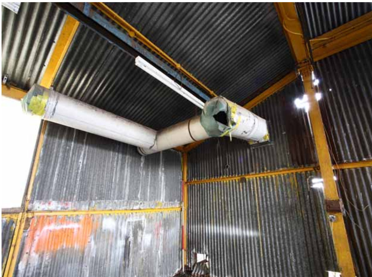
Plate 36: Heating ducting in the north-west corner of Room 1 that passes into the brick outshut
