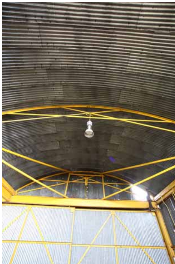
Plate 33: View of timber bracing to the truss of the southern barrel vaulted roof
