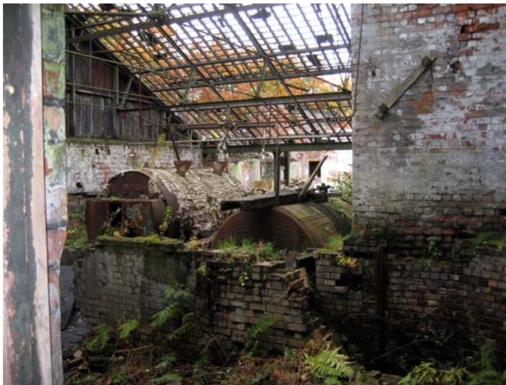
Plate 19: Looking north through the Boiler House Building 8, showing main flue and putative economiser housing in the foreground
