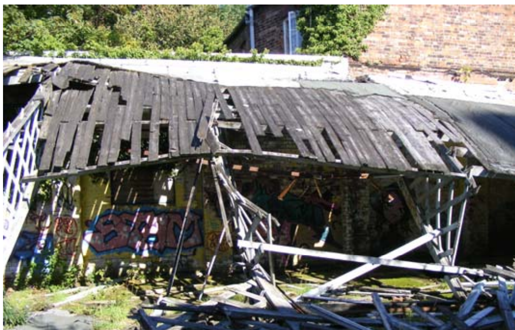
Plate 26: The collapsed roof of Building 19 in 2007, immediately prior to the survey
