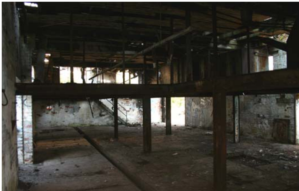
Plate 13: North-facing-view of the interior of Building 4, detailing the steel mezzanine floor and iron tanks
