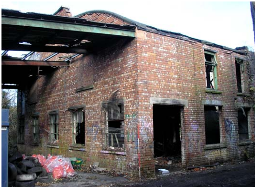
Plate 11: North-east-facing view of the south elevation of Building 3. The adjacent corrugated iron and steel shed (Building 2) is visible on the left.
