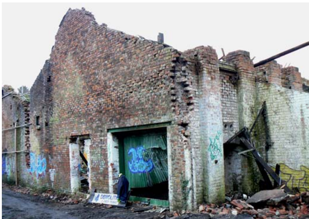
Plate 21: North-facing elevation of Building 13, showing ventilator-pattern brickwork. Note the pair of guide eyes built into east-facing elevation, providing access from Singe House
