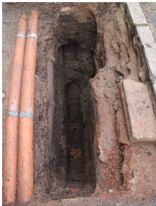
Plate 2: Trench 2, facing west, with large cuts for service pipes, and the concrete raft which extends beneath the road
