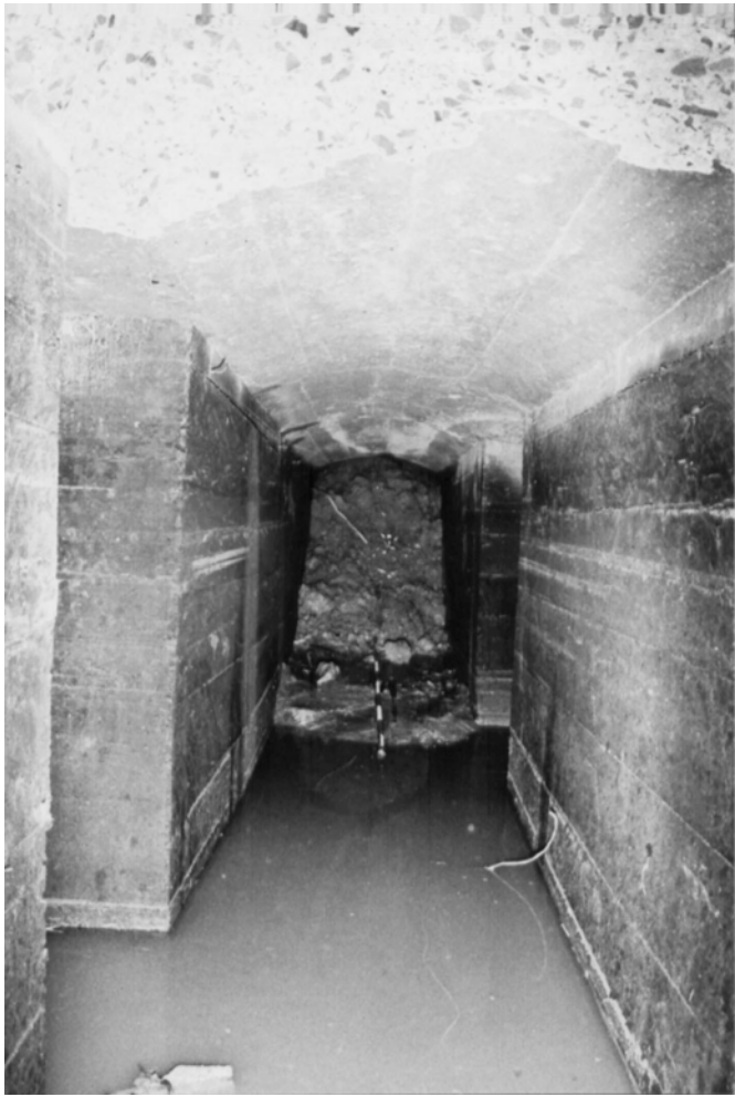
Plate 6: Blocked tunnel B3, looking south
