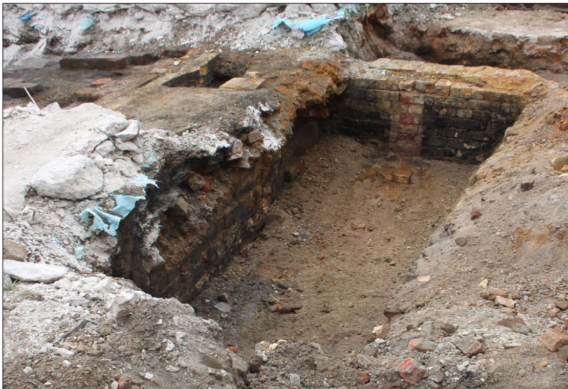
Plate 14: Southern boiler bay, looking west with northern elevation of southern wall of boiler bay to left and Trench 3 extending south beyond it
