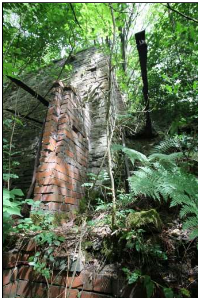
Plate 57: Corner of stone-built revetment wall, with redundant roof beam extend to right of centre
