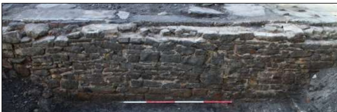
Plate 15: The north-eastern exterior elevation of the Phase 1 wall defining the southern bay of the mill/bleach works
