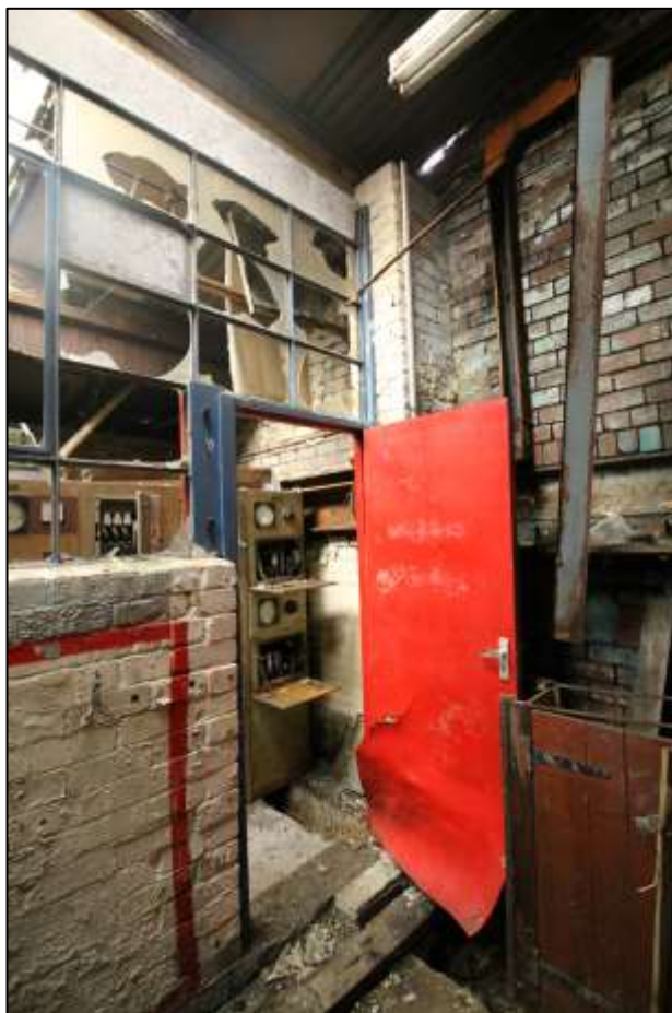
Plate 52: Electrical generation equipment at southern end of the eastern wall of the larger cell, facing south-west
