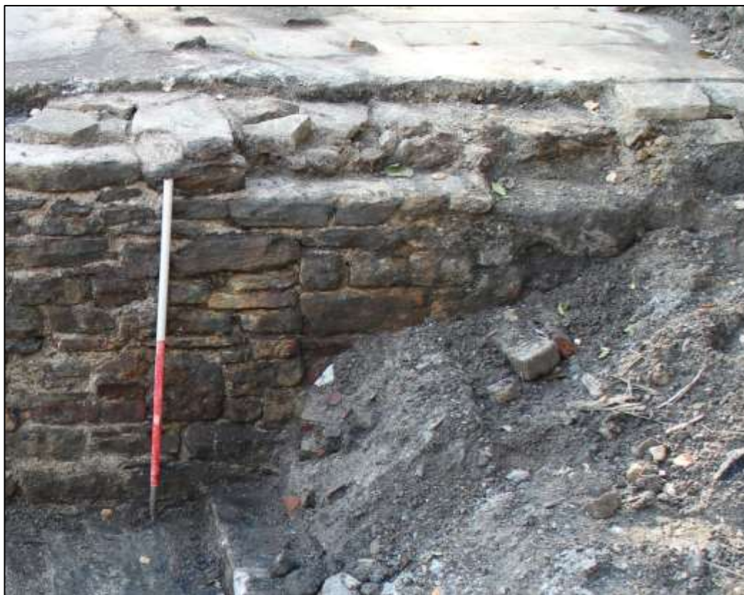
Plate 18: Infilled masonry (right) in the Phase 1 wall defining the southern bay of the mill/bleach works
