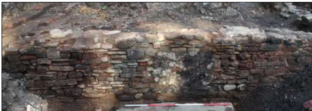
Plate 14: The south-western exterior elevation of the Phase 1 wall defining the northern bay ( Room 1017 ) of the mill/bleach works
