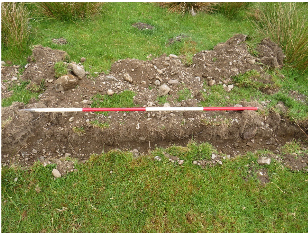
Plate 5: Section of the cable trench in Area 5, viewed facing east (scale 2m)
