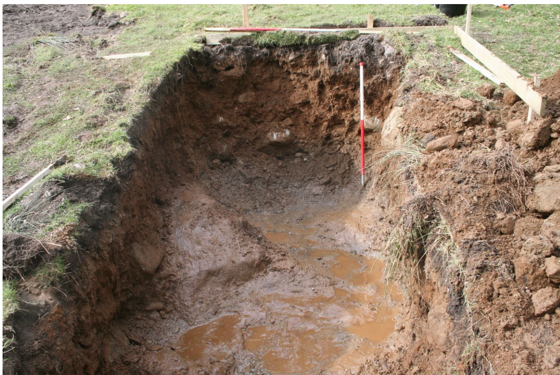
Plate 3: General shot of excavations for the Powerhouse, viewed facing west (scale 1 x 1m)
