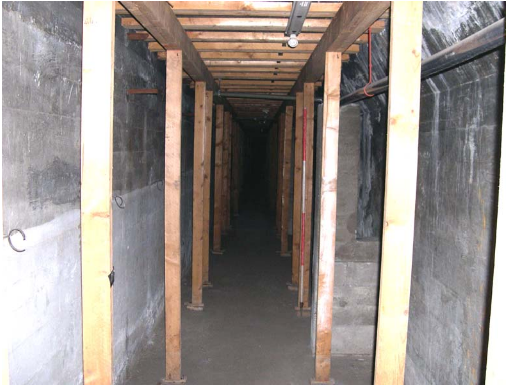
Plate 28: General view of part of the west side of the basement of the baths
