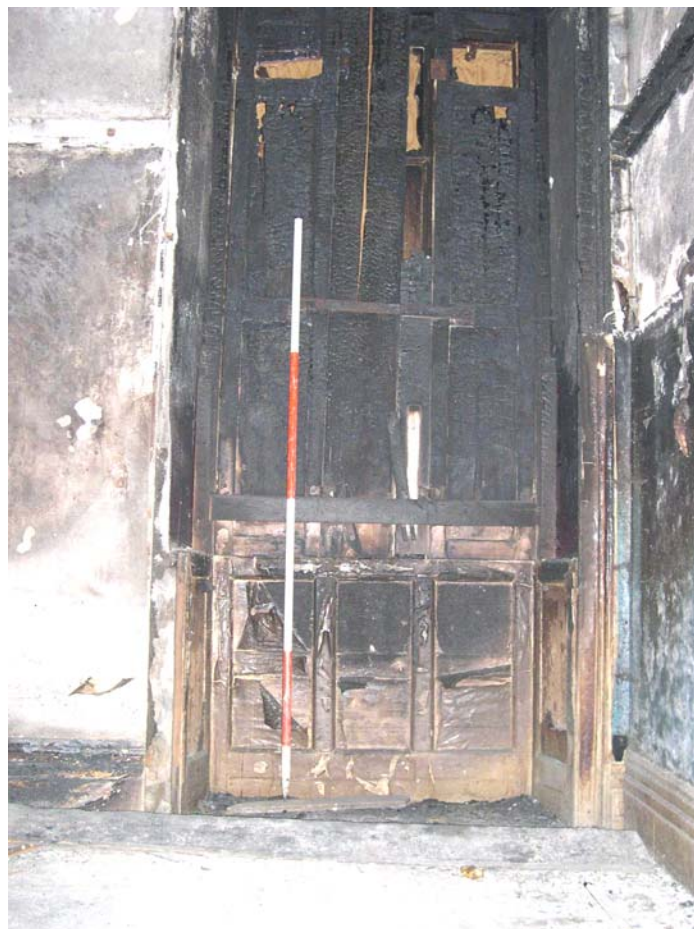
Plate 14: Window in Room 7 of east Bridge House, showing remains of badly damaged shutters and surrounds
