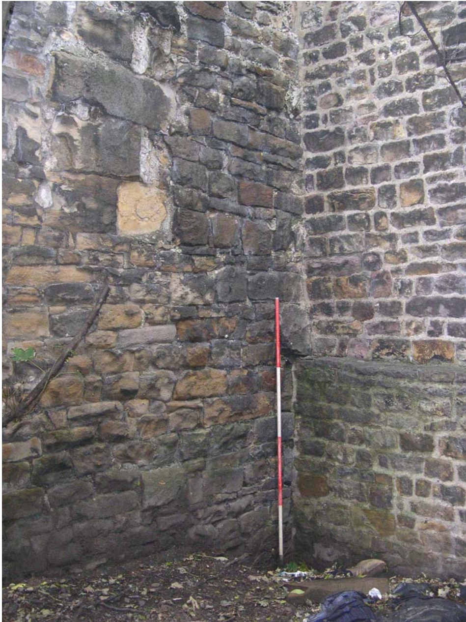
Plate 10: Detail of the junction between the east link wall and east Bridge House
