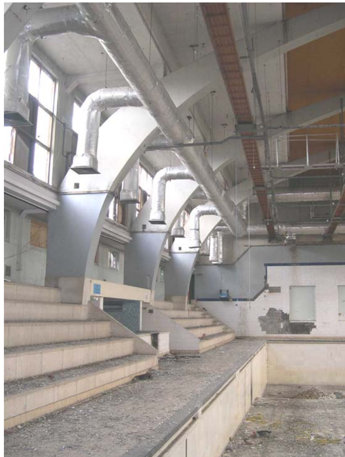
Plate 35: Detail of pre-cast concrete portal frames on east side of main pool (Room 19 ), baths
