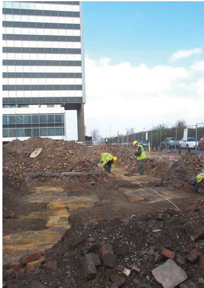
Plate 6: Working shot of wall foundations, showing walls 704 (background), 705 , and 706 (foreground), viewed from the south-east
