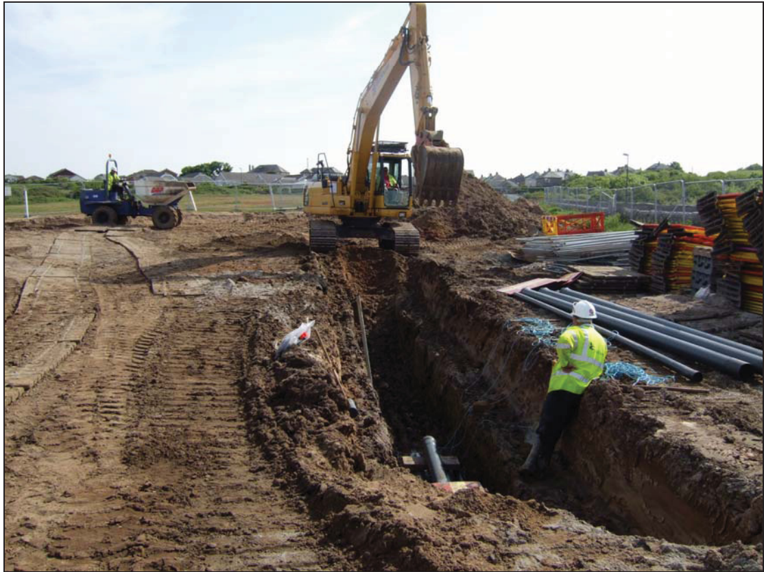
Plate 7: Excavation of trench for cable duct in land adjacent to Old Smithy Lane, looking north-west
