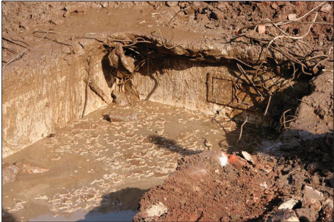
Plate 9: Detail of the exposed metal hatch covering access to the ventilation shaft (© Duncan Davis)
