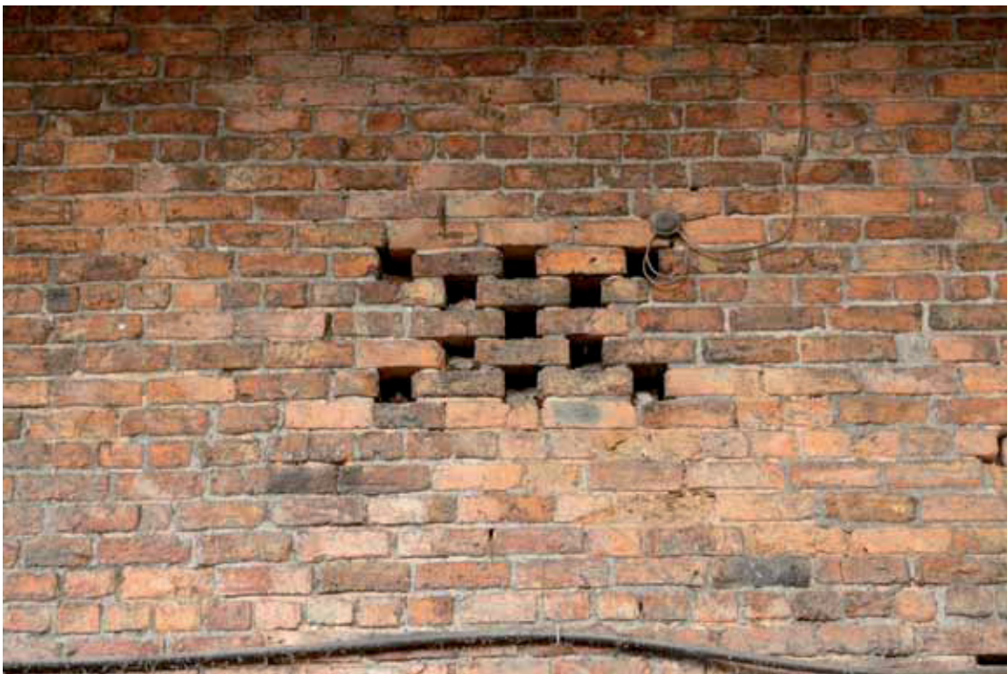
Plate 25: Detail of geometric style brick vent within the rear wall of Building 1
