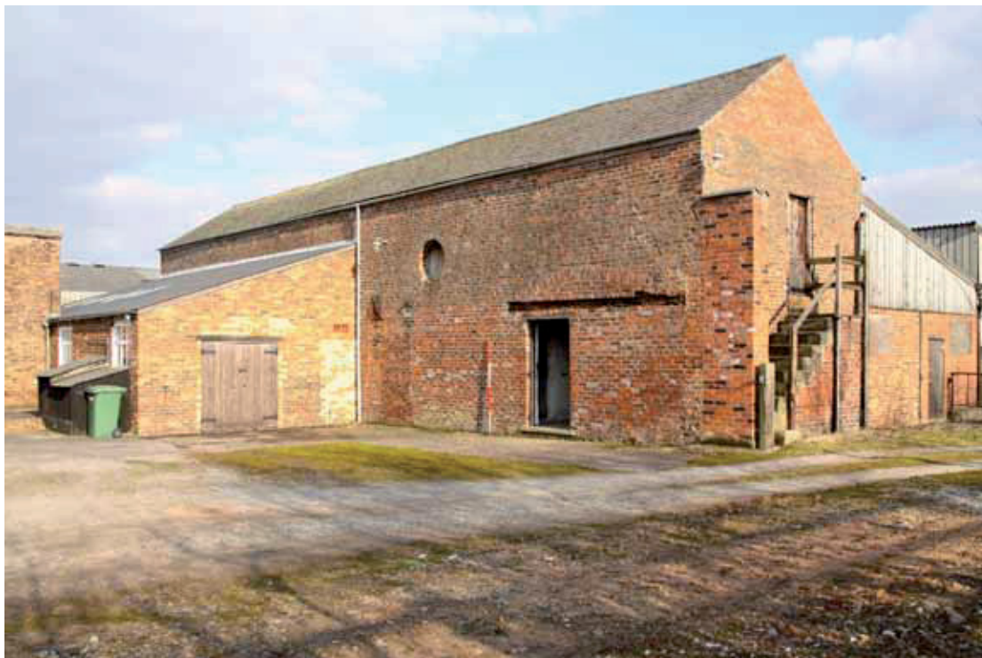
Plate 22: The front elevation of the barn. The relieving arch for the wagon door is evident above the timber lintel
