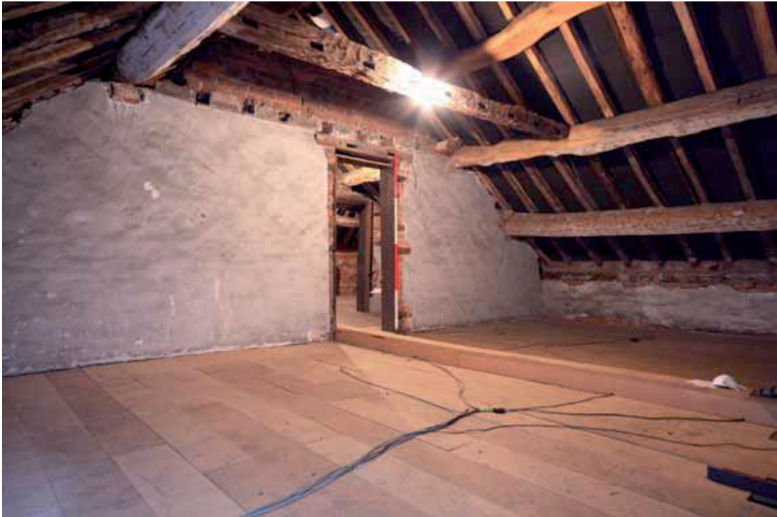
Plate 11: Attic space showing sockets for ceiling joists within the tie-beam and brickwork
