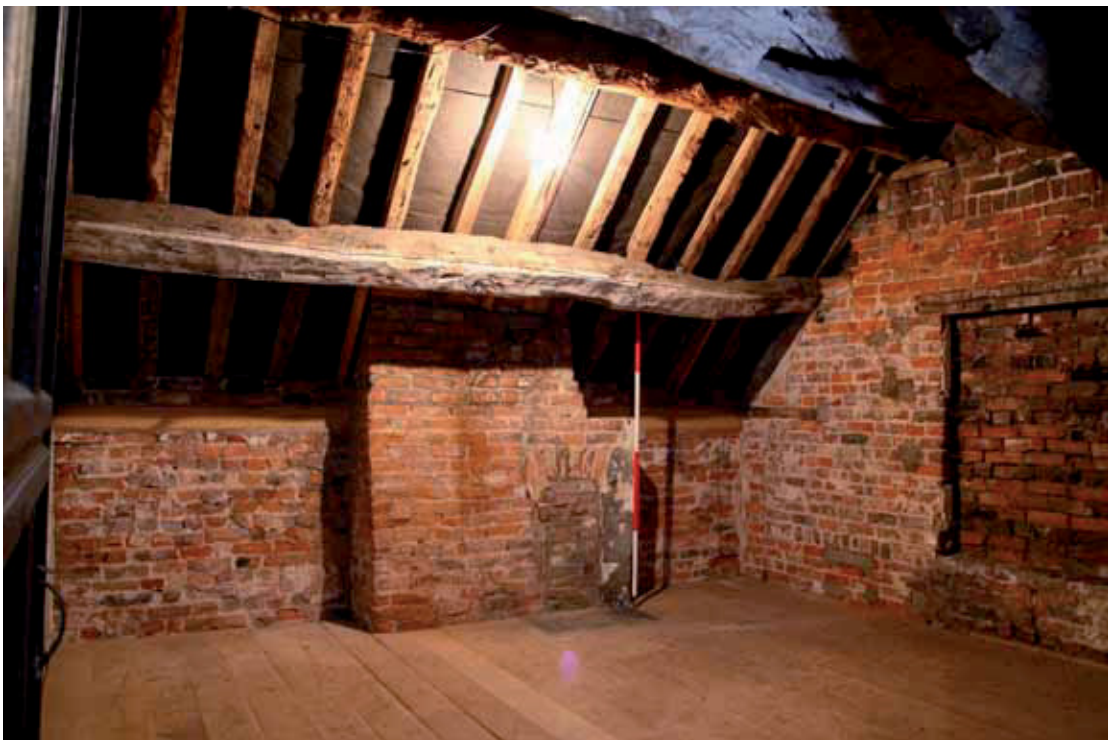
Plate 14: Blocked fireplace and blocked window in the attic
