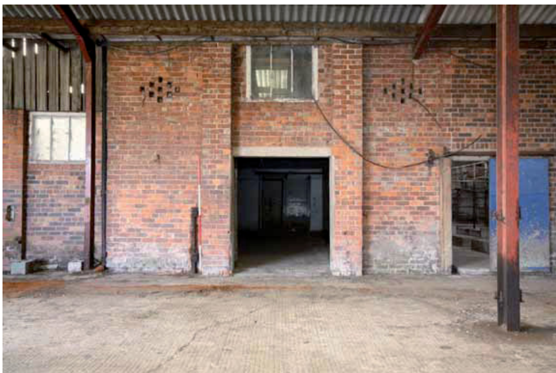
Plate 23: Gable end of the barn (Building 1), now internal, showing re-built face with Building 3 keyed in on the right
