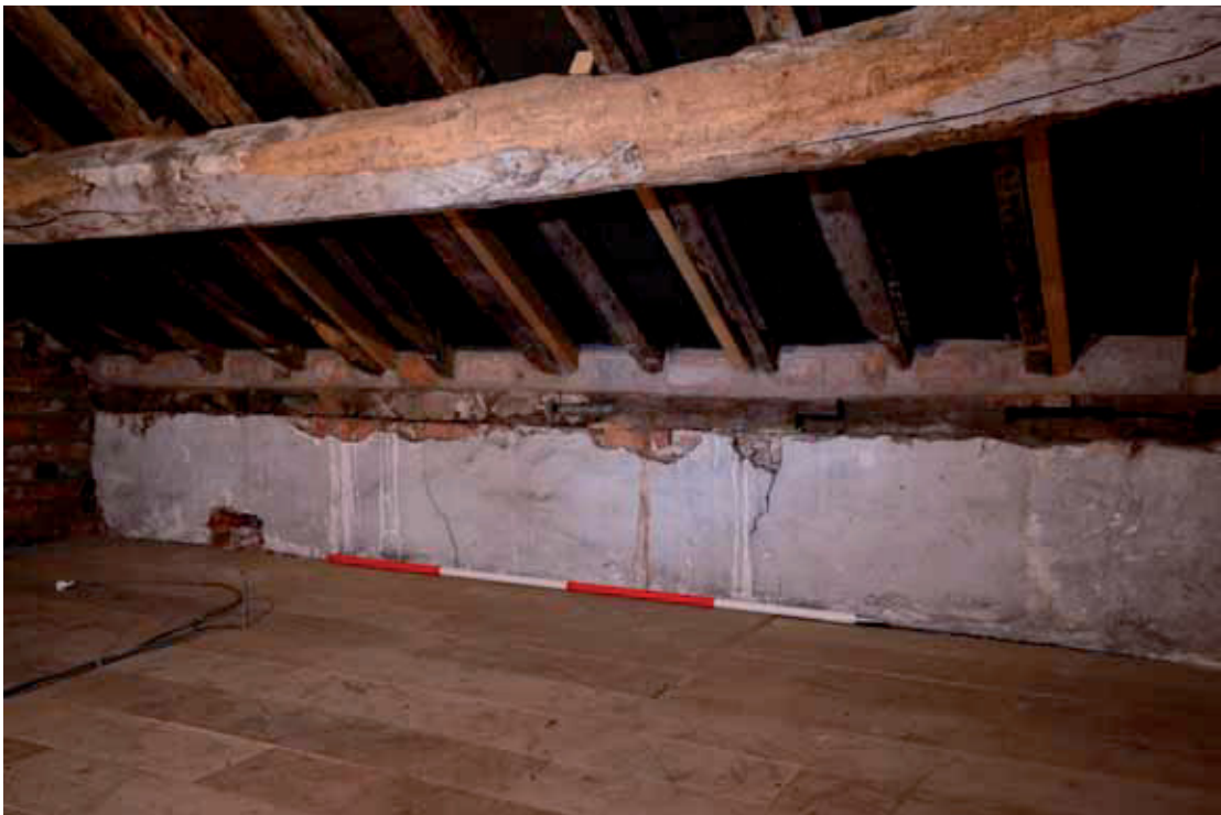
Plate 12: Detail of wall plate with edge-halved, scarf joints, and new brickwork above
