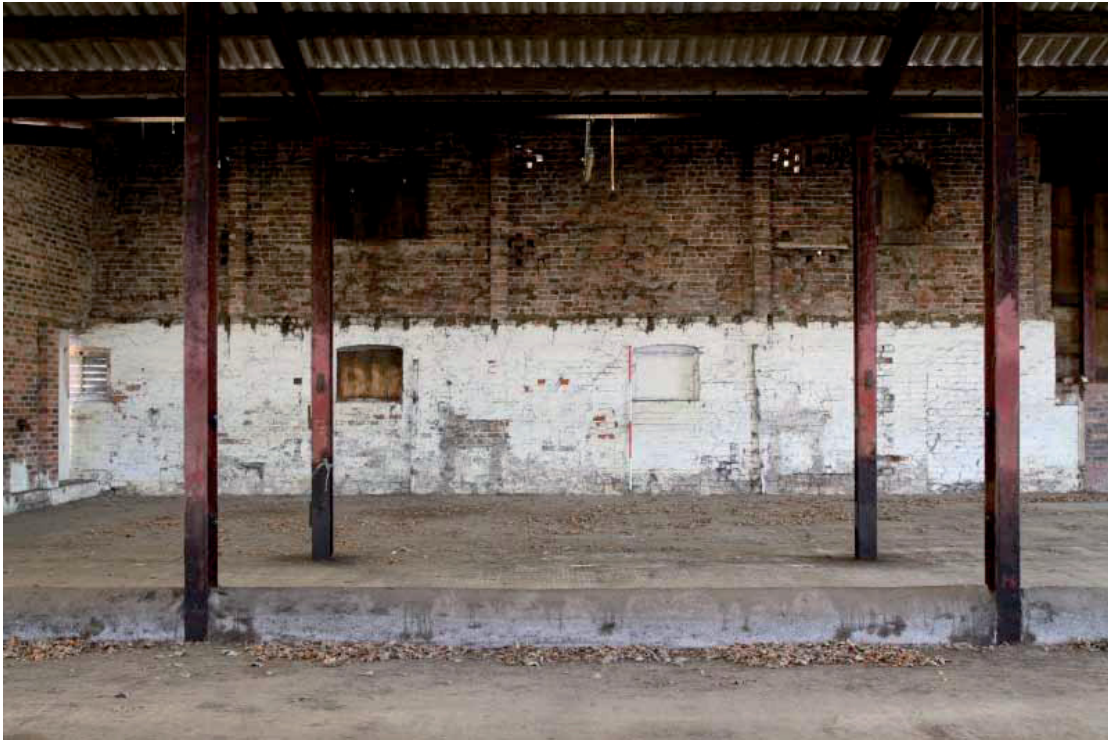
Plate 32: Internal elevation of Building 2 within Building 6, showing the sockets for the floor joists
