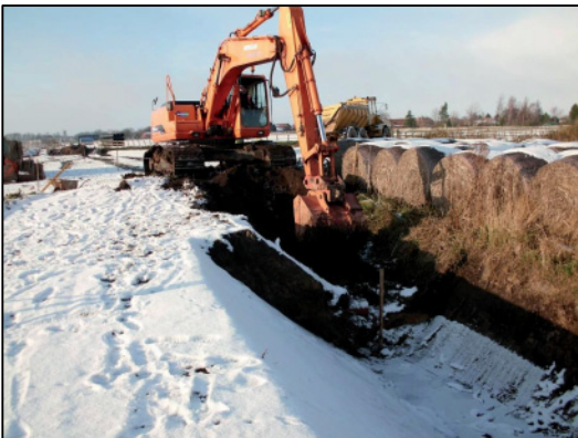
Plate 9: Working shot in the Trench 3 area, looking north-west from the west end of the Zone 2 works.
