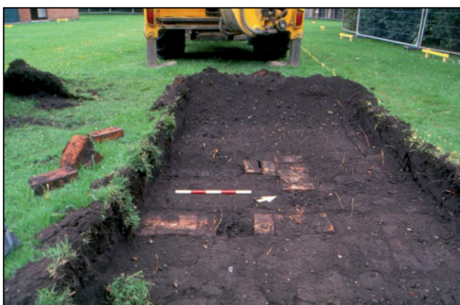
Plate 5: Structure 1 exposed in the strip of the new park management building footprint, looking north-west.
