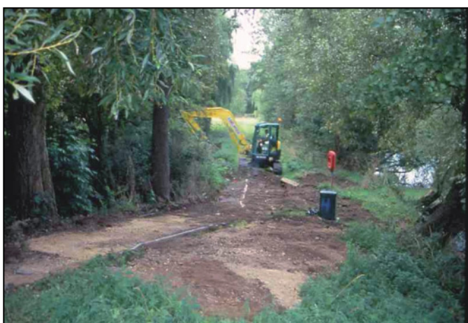
Plate 7: Working shot during path stripping in Area A, looking south from near the Farndon Road bridge.
