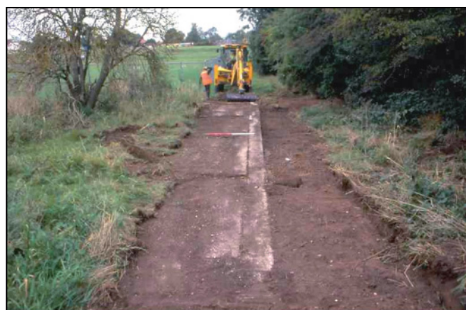
Plate 9: The WW II concrete structure encountered during path stripping in Area D, looking north-east.
