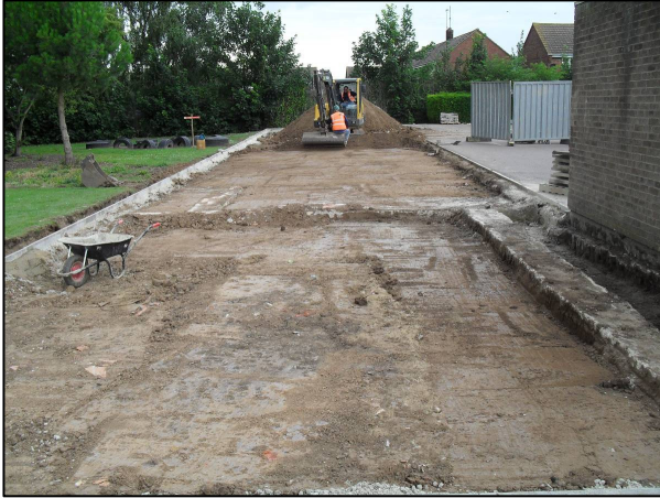
Plate 7: Area 2 at the end of stripping the playground extension footprint, looking north. Structure [202] and the area of modern infill can be seen in the foreground.
