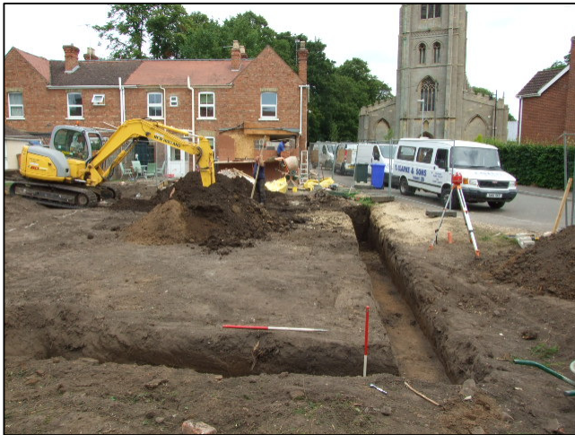
Plate 1: General shot of the site during the groundworks, looking north-east from its south-eastern corner.
