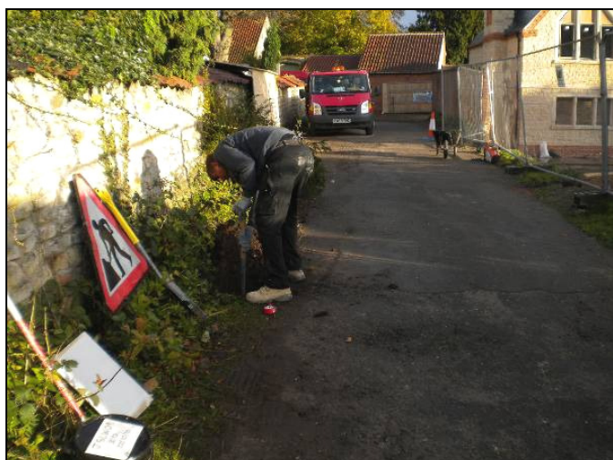
Plate 11: Excavation of a test pit at the western edge of James Street, looking north towards the new building.
