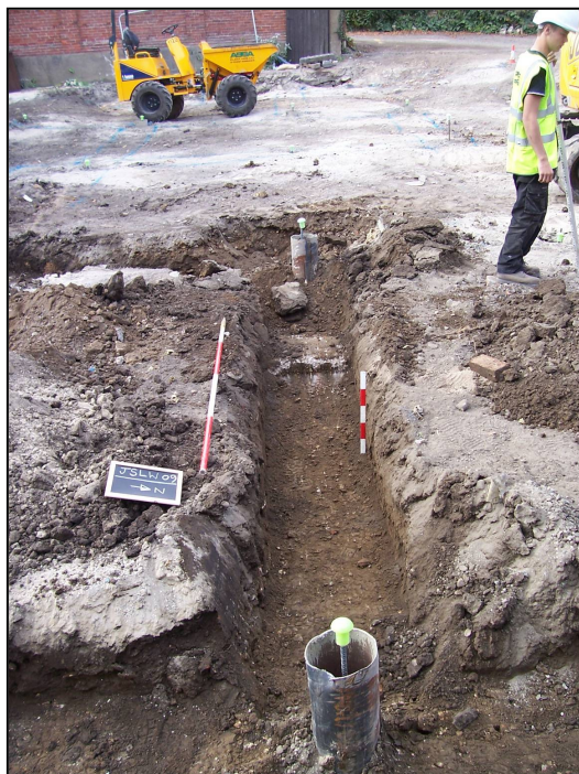
Plate 4: Excavation of the ground beam slots for the new building, following the installation of the piles (foreground and centre), looking west.
