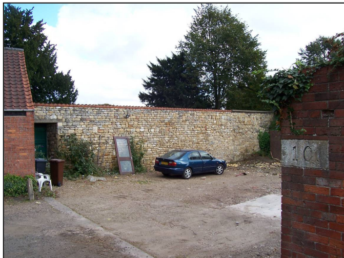
Plate 1: General shot of the north side of the site post-demolition, looking north-east from the James Street entrance towards the scheduled boundary wall.
