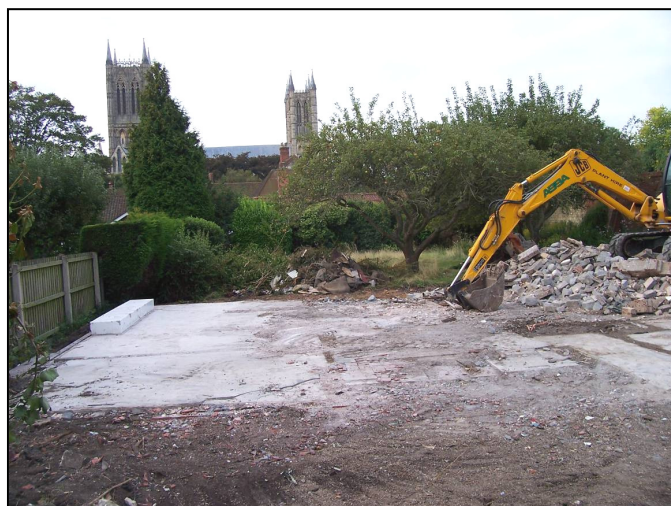
Plate 2: Removing the concrete floor slab of the demolished bungalow, looking south towards Lincoln Cathedral.
