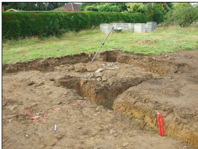
Plate 6: The footings trenches during excavation, looking south from the centre of the house plot.
