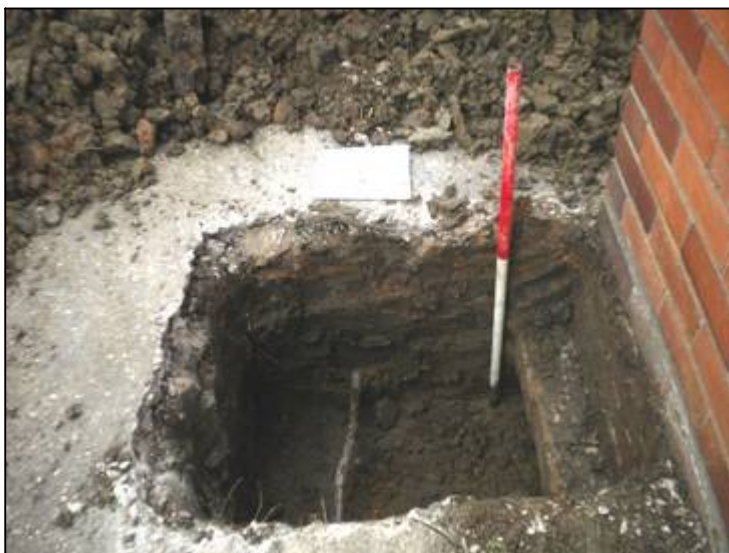
Pl. 3 Ground beside the existing house had been disturbed by the original foundation trench and by an adjacent water pipe trench (looking north at the north-west corner of the house, scale 1m).
