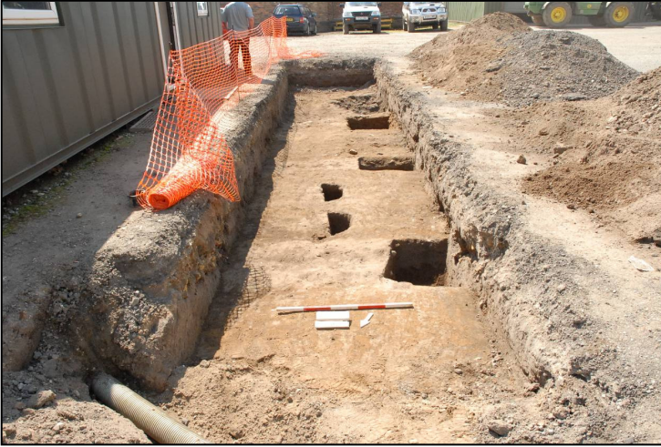
Plate 10: General shot of Trench 5 post-excitation, looking S, showing its position relative to the temporary farmyard building.
