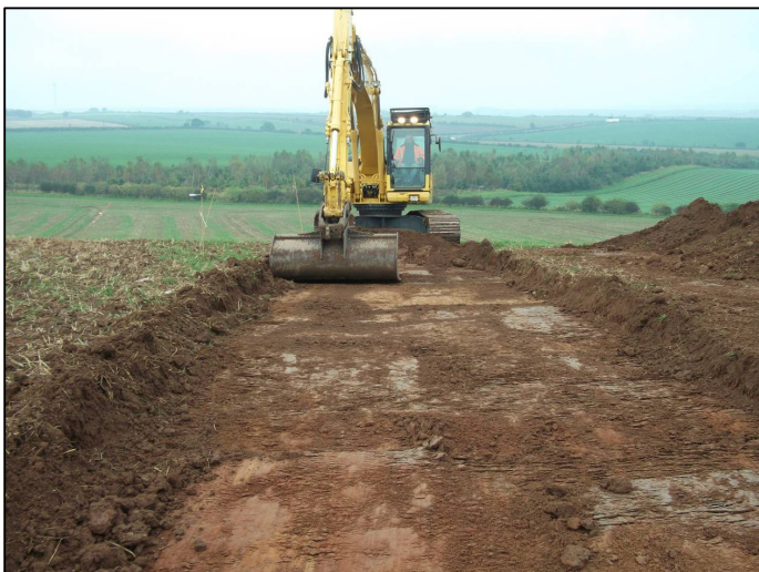
Plate 1: General shot during the machining of the W end of the access road, looking W, showing the position of the site, raised above the surrounding landscape.
