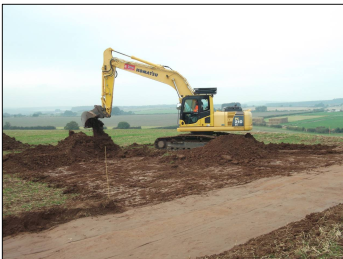
Plate 2: Machine-stripping of the hard-standing area around the pylon base, looking SW, showing the exposed subsoil 1001.
