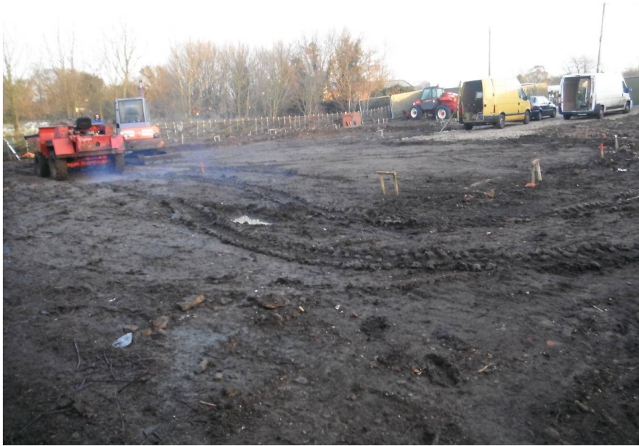
Plate 1: General site shot looking north.
