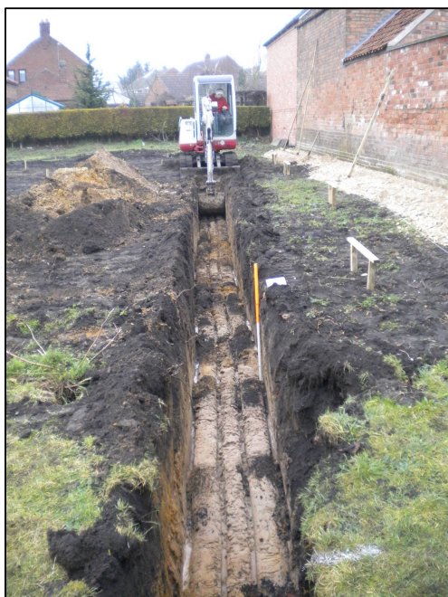
Plate 2: Working shot during the excavation of foundation trenches in Plot 2, looking W.
