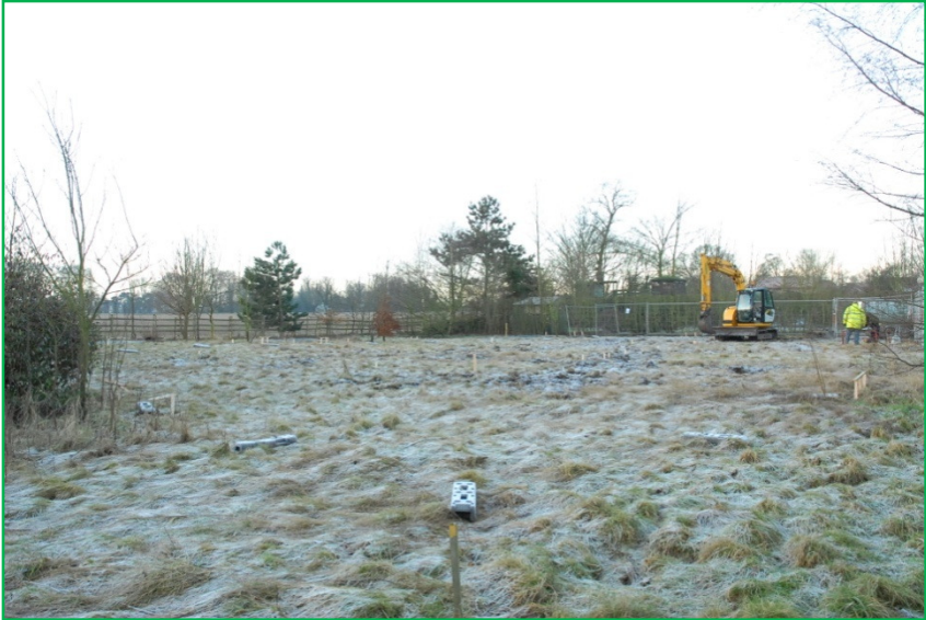
Plate 1: Site shot, looking southwest across the area for the house plot showing the beginning of stripping for the access road.
