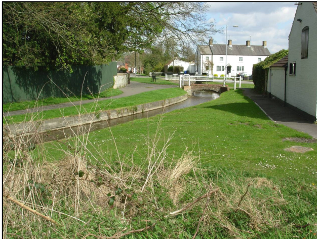
Plate 8: The Dunholme Beck, looking E from the E edge of the site, showing the concrete culvert in which it runs.
