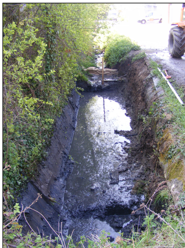
Plate 3: General view of the ditch after the works were completed, looking south.
