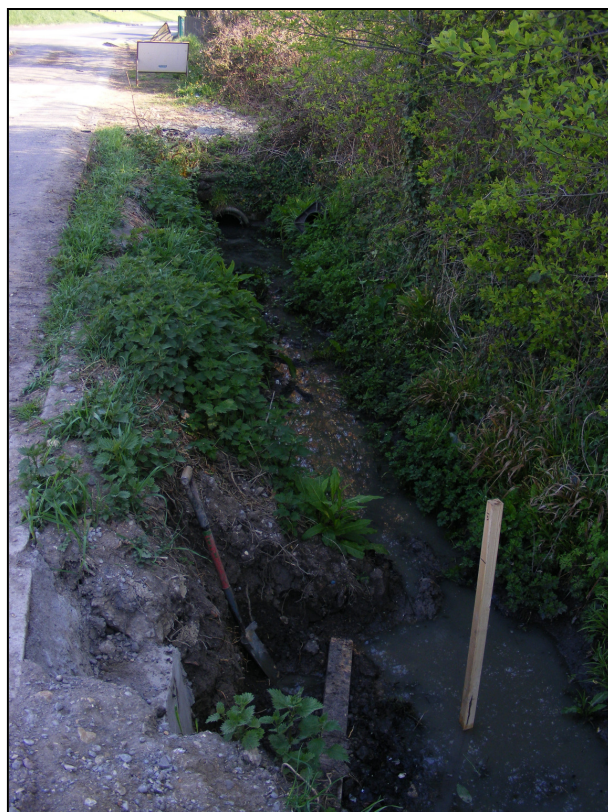
Plate 2: General view of the ditch before the works were undertaken, looking north.
