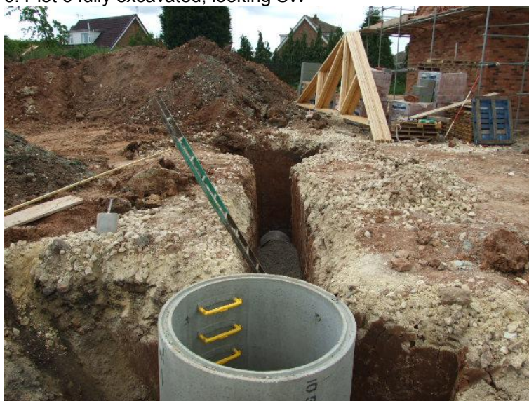
7. Drainage runs SW09 and SW10 in the central part of the site, looking east
