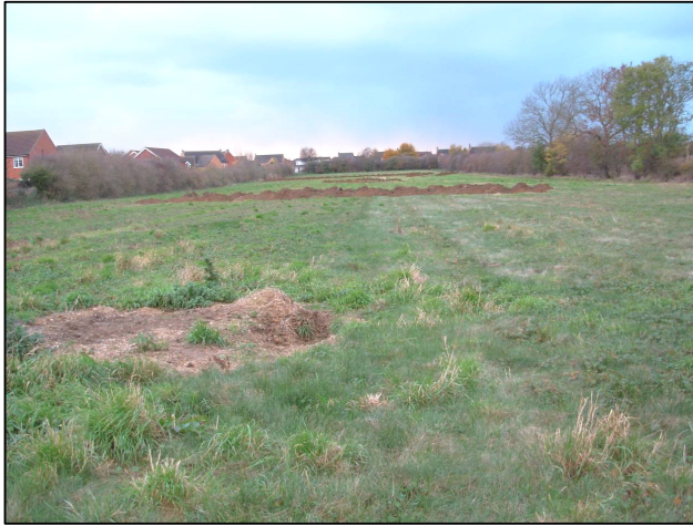
Plate 1: General shot of the site after machine excavation of the trenches, looking W from the E end of the site.
