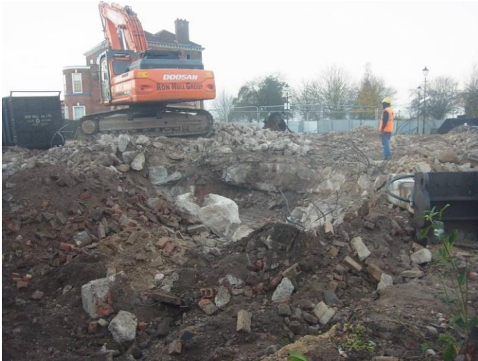
Plate 1: Site on arrival. Concrete foundations just visible beneath rubble of demolished buildings. Looking SW
