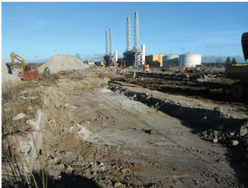
4. General view of the south-western part of the site prior to foundation removal, looking east
