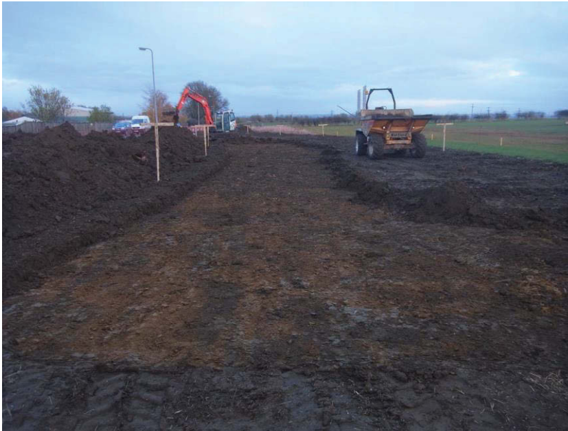
1. Topsoil stripping for the new access road, c. 500m west of the monitoring area, looking east
