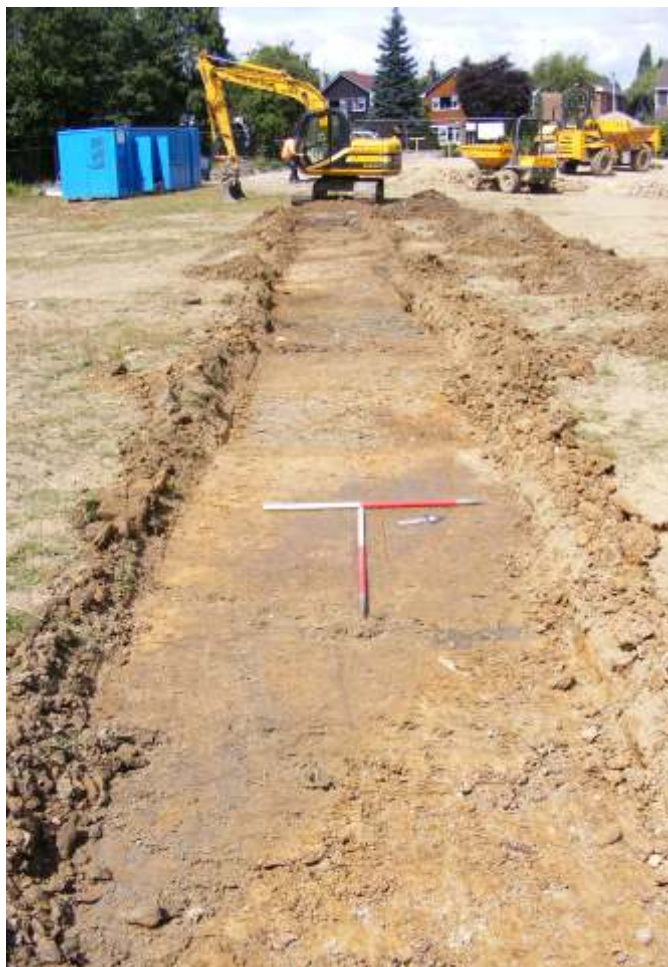
Plate 8: Trench 11 after excavation, looking west north-west. Ditch [1102] can be seen in the foreground, with land drains in the middle of the trench.
