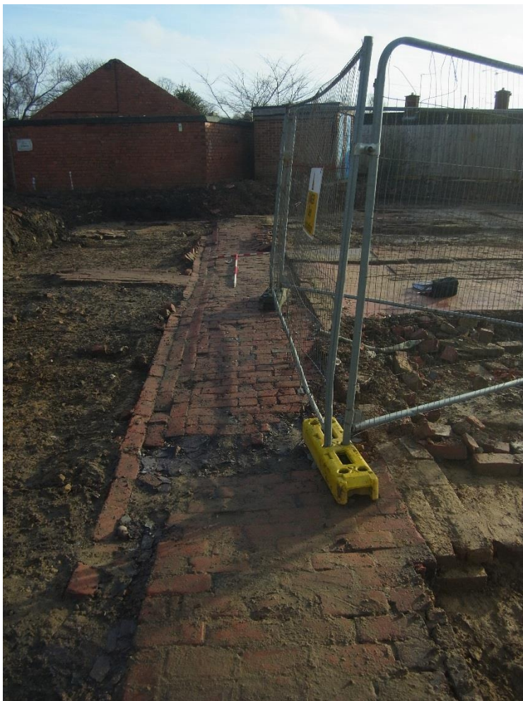
14. Pathway 141 (NW-SE) running parallel to NW-SE extent of Glue and Leatherworks. Looking SE.
