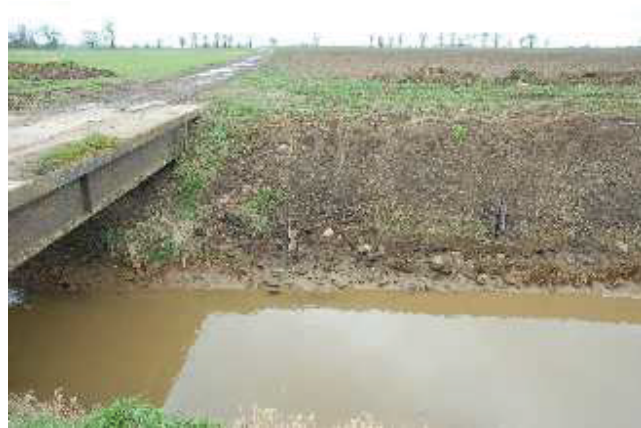
Plate 8: The remains of Bridge B7 can be made out, but the current road follows the course of an earlier trackway
