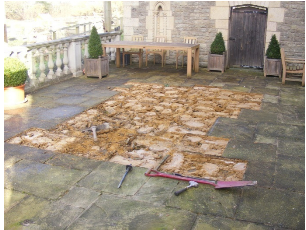
Plate 2 – Patio slabs lifted (looking north).
