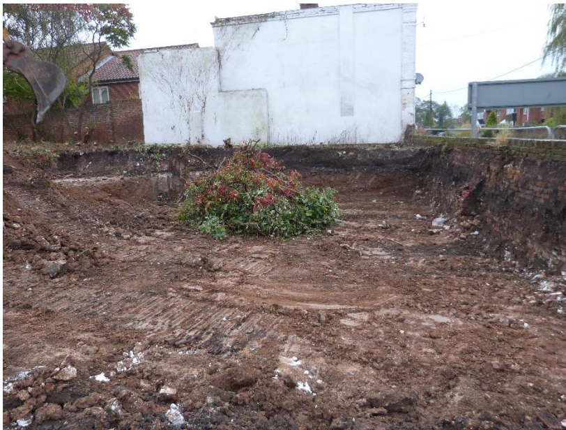
6. Ground works carried out the day before archaeological monitoring was recalled, looking east
