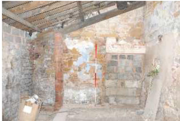
Plate 5: The internal walls of the lace-making cottages remained standing, but the internal doorway has been boarded up.
