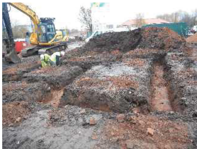
Plate 9: Plot 9 after excavation of the footings. The layer of demolition rubble (1022) was especially prevalent at this location.
