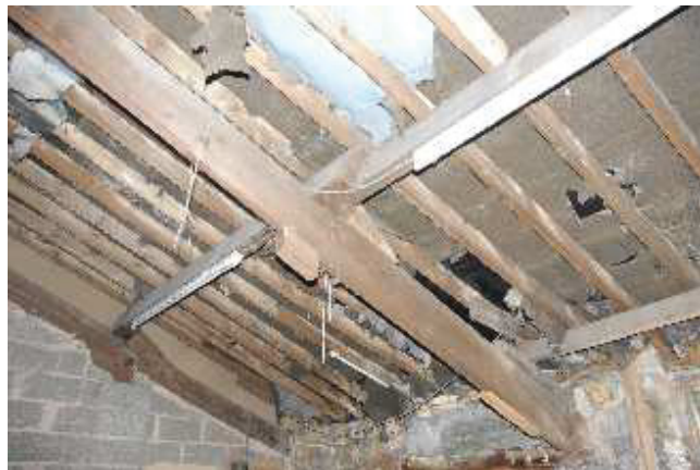
Plate 6: The roof of the central section of the lace-making cottages. Most of the structure remained, understandably in a state of disrepair.
