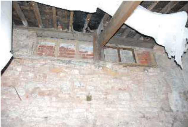
Plate 4: The central section of the 19 th century lace-making cottages, as seen from the inside. The windows have been boarded up by modern bricks, but their form is clearly defined.
