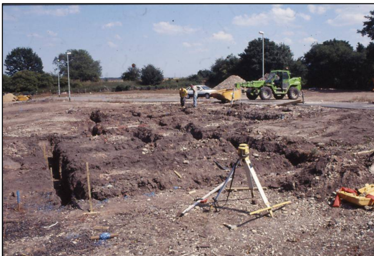
Plate 3 (left): General view of the completed footings trenches for plot 1, looking east.
