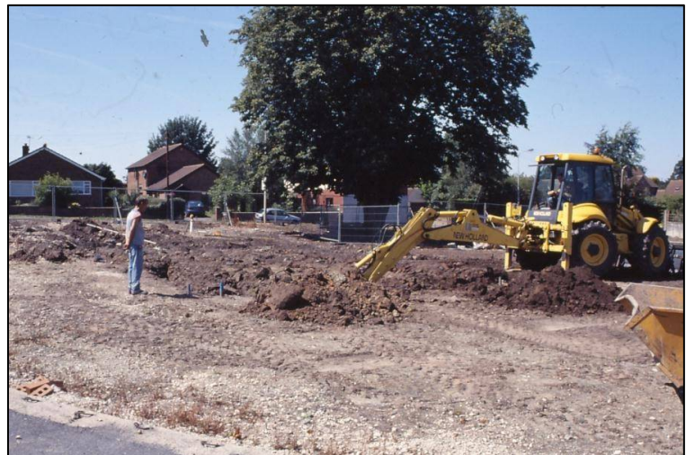
Plate 2 (right): General view of the site during the machining of plot 1, looking northwest.
