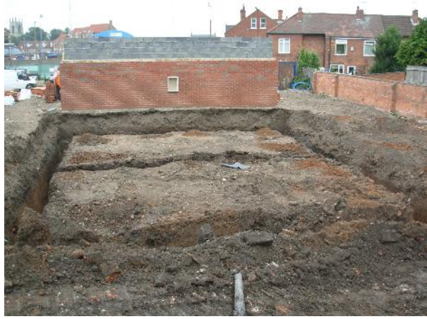
Plate 5: Plots 12-13 after completion, looking south-west. The wall 404 was located in the bottom right corner of the photograph
