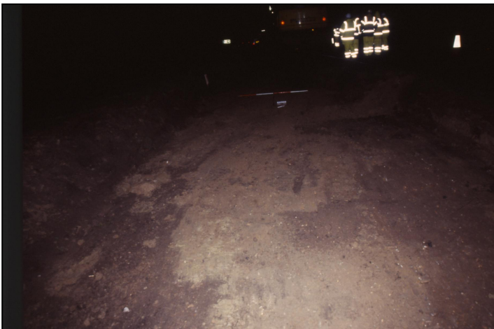
Plate 2 (right): General view of the stripped area of the layby from ch. 55 – 75 showing the exposed layer (002), looking northwest.
