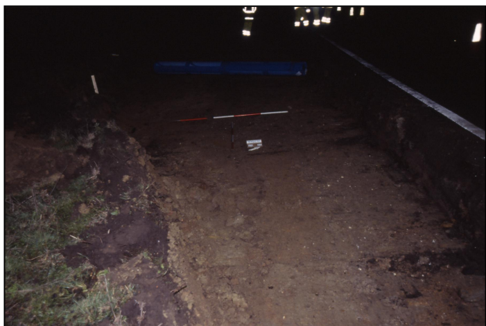
Plate 3 (left): General view of the stripped area of the layby from ch. 35 – 55 showing the exposed layer (002), looking northwest.
